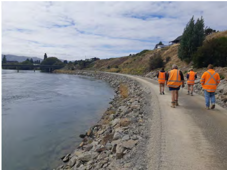
Figure 2 River channel asset, Albert Town (Clutha River/ Mata-Au) Rock Buttress flood repair works completed in February 2021.
