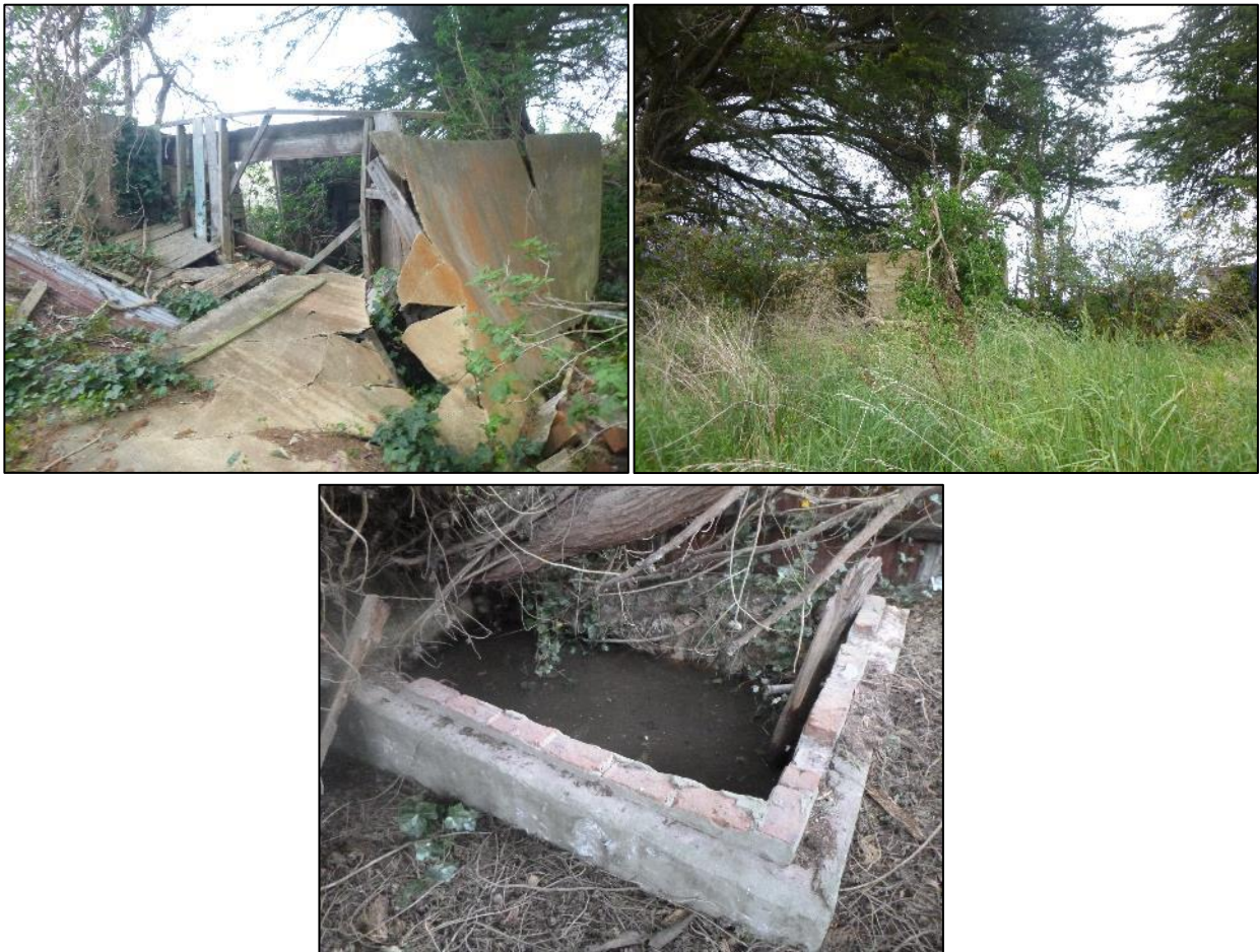
Figure 5-185-48 Current condition of the homestead structure with the ceiling collapsed and walls listing heavily, looking north (top left) Structure barely visible through thick vegetation, looking south (top right) and the current state of brick and concrete lined structure looking north (bottom).
