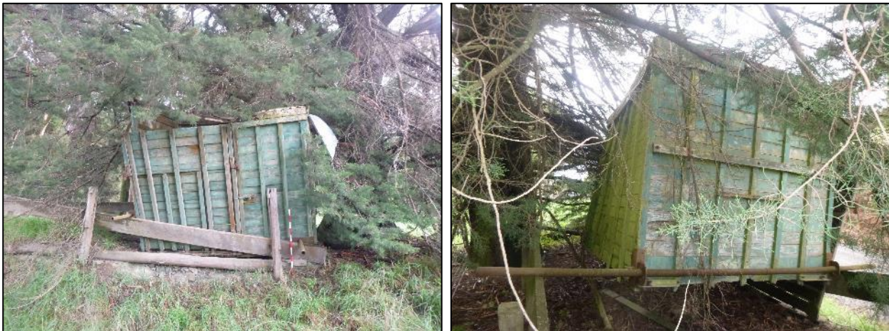
Figure 5-465-43 Horse float. Note that the roof would normally be flat however the structure is damaged causing the roof to sag in the centre of the side facing the road (left) but remain relatively flat at the opposite side (right). The nails used for the construction of the structure and associated fences appear to be modern.
