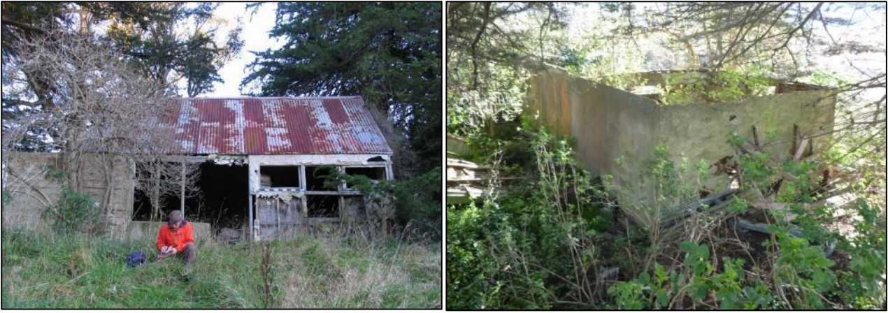
Figure 5-165-16. Photograph taken looking south in 2009 (Jacomb, 2009) and northwest in 2017 showing the deteriorating condition of the site (Mitchell, 2017).
