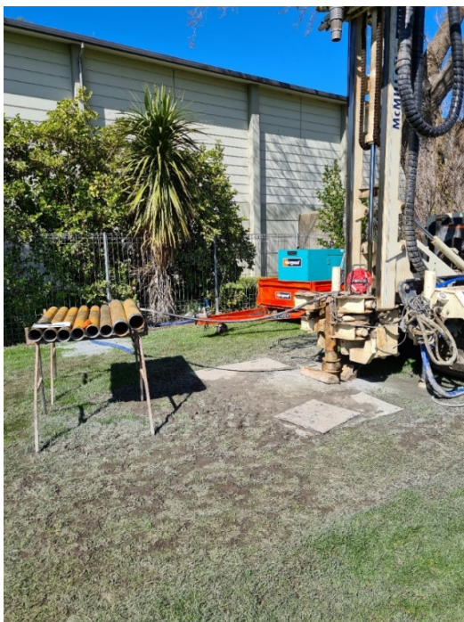
Figure 4: Drilling rig set up for aquifer testing in South Dunedin (Tonga Park, October 2021)
