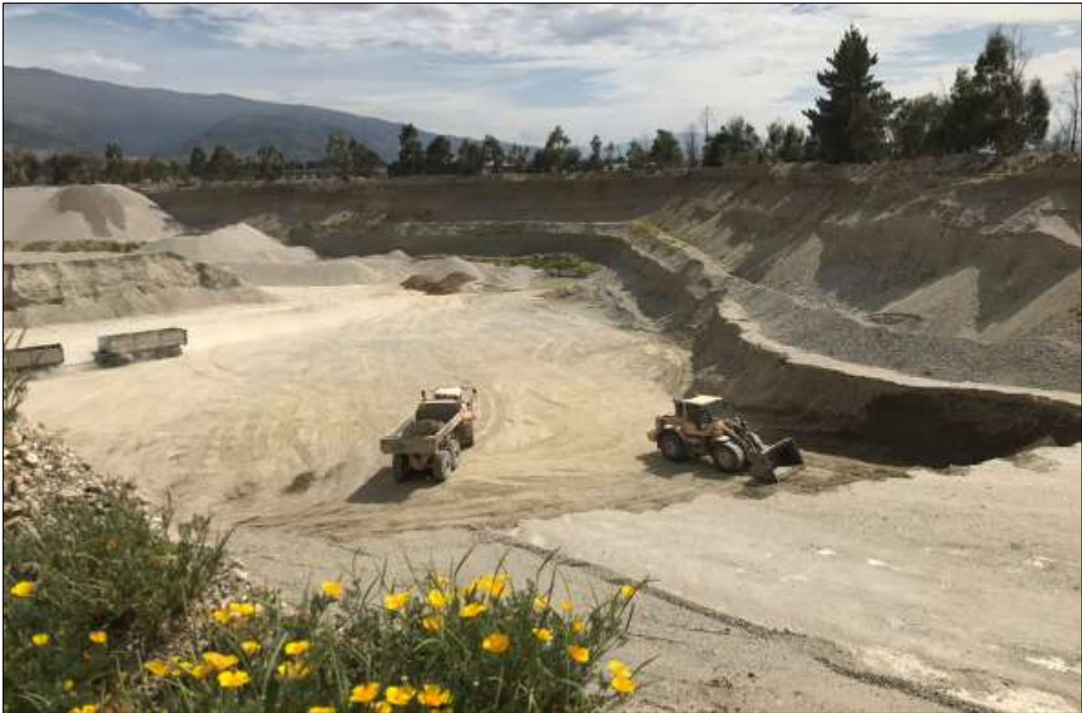
Figure 4: Photo of loader and trucks working on the quarry face (Source: Beca Dust Assessment 21/1/2020)
