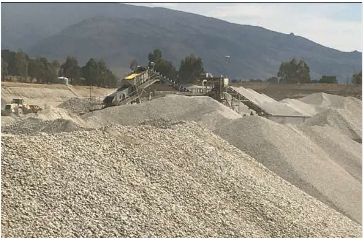
Figure 5: Photograph of screening and washing plant with washed aggregate in the foreground (Source: Beca Dust Assessment 21/1/2020)
