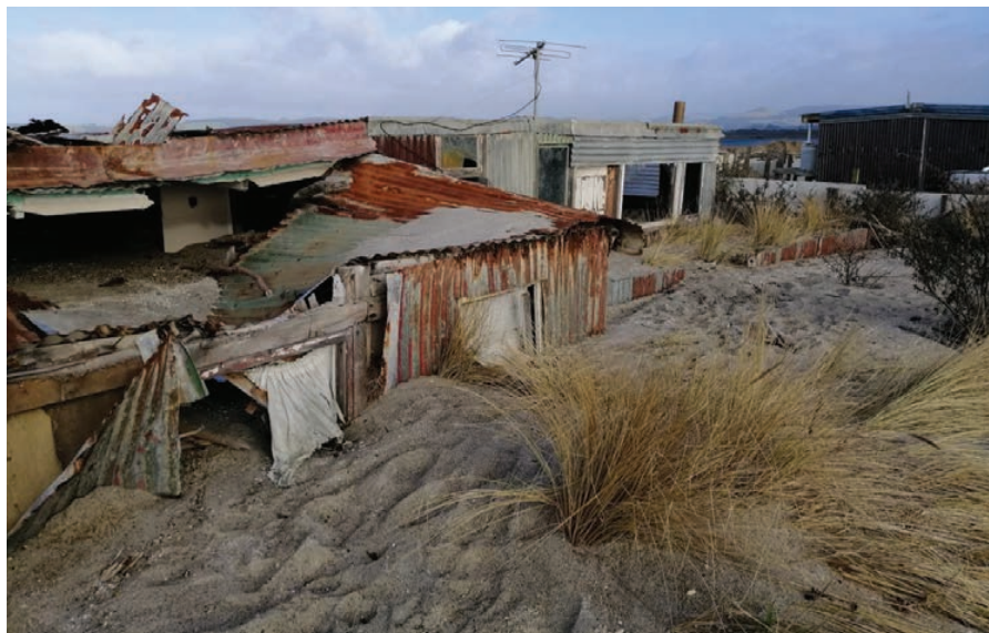
Figure 2.14: Evidence of wave overtopping south of the Koau Mouth southern training wall (Jacobs, 2020).
