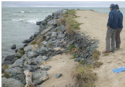
Figure 2.8: Koau River Mouth training wall (north) following a storm when it was badly damaged by the removal of rip rap by high sea levels and large waves, exposing the training line to further damage (Bloor, 2017).
