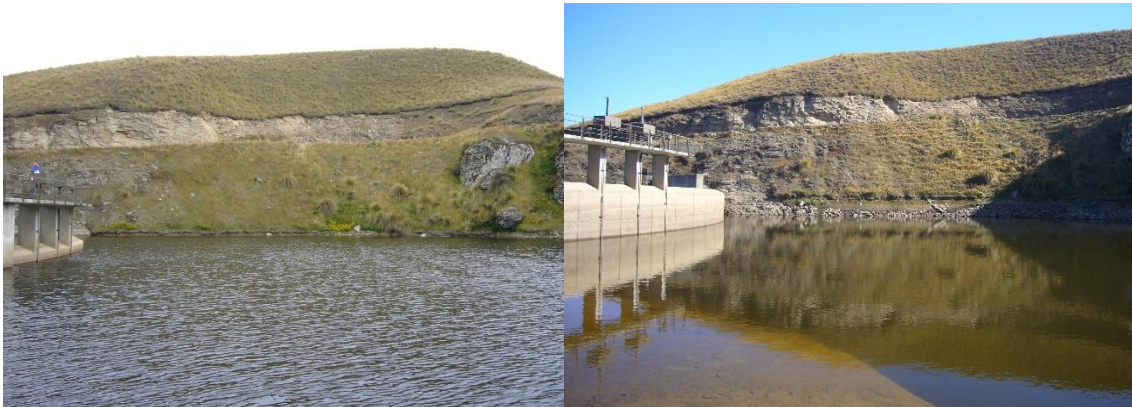
Figure 4: Onslow dam with lake levels close to capacity (left) and 2-2.5 m below crest (right)
