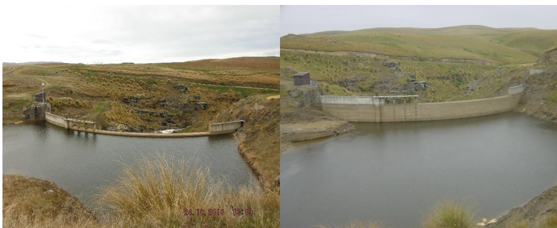
Figure 3: Lake Onslow Dam at high lake levels (left) and lake levels 4.35 m below crest (right)
