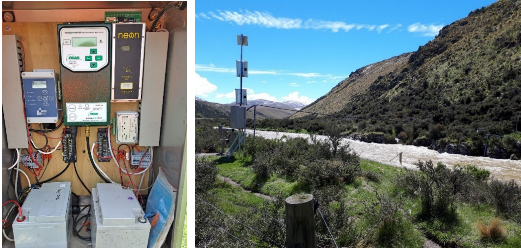
Fig.2: Left: An ORC logger box containing two completely independent telemetry systems for a flood warning network site. The blue HyQuest iRIS logger on the left communicates data from a bubbler water level sensor (green box in the middle – see text below for further information) via a cell phone network, while the dark grey NIWA NEON logger is a satellite device that is connected to a bridge mounted radar. Both systems have independent solar power supplies and back-up batteries.
