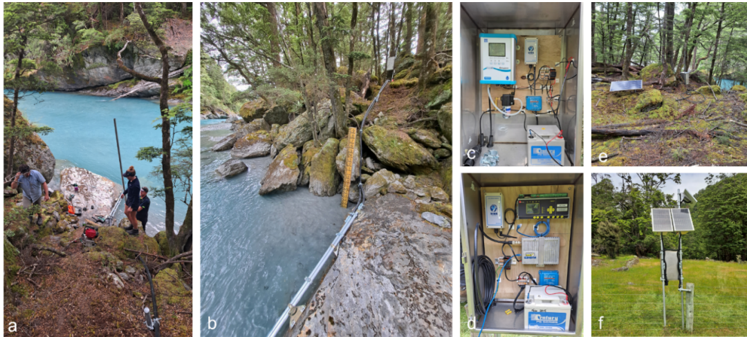
Fig. 5: Example of recently installed new flow site on the Rees River at Invincible that will provide better flood warning for the community in Glenorchy. a. installation in progress by Emily Olson, Jono Young, Tim Harrex, Nick Boyens (not in picture). b. completed river installation. The instruments are submerged into the river through the steel tube that is anchored to the rock. The site has no cell phone reception and too much bush coverage to obtain good satellite coverage. Thus the team has installed the new NIWA LoRA IoT links to transmit multiple signals from the water level sensor site (c. and e.) in the bush to the logger and satellite modem out in the open (d. and f.).
