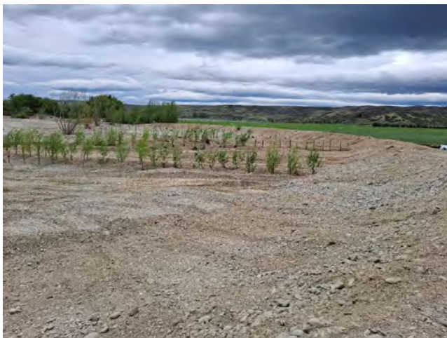
Figure 5 Manuherekia River, Leasks Bend after realignment and commencement of planting of willows.
