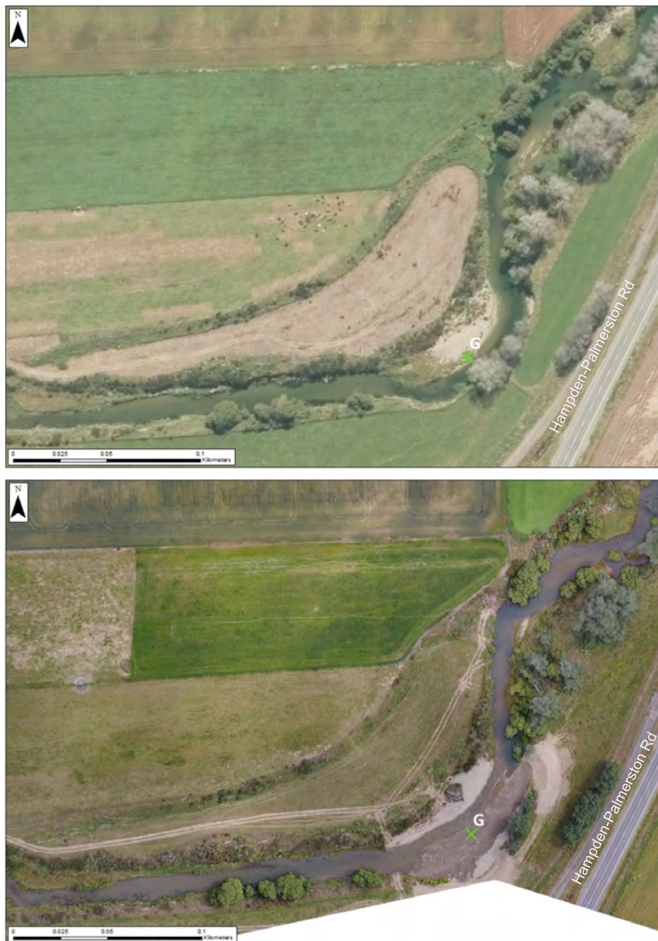
Figure 22. Comparison pictures of operation location G. Upper image before works completed (Aerial imagery 2014), lower image after works completed (Aerial imagery 2016), the gravel beach has been removed, the channel realigned and bank protection measures out in place on the true right.
