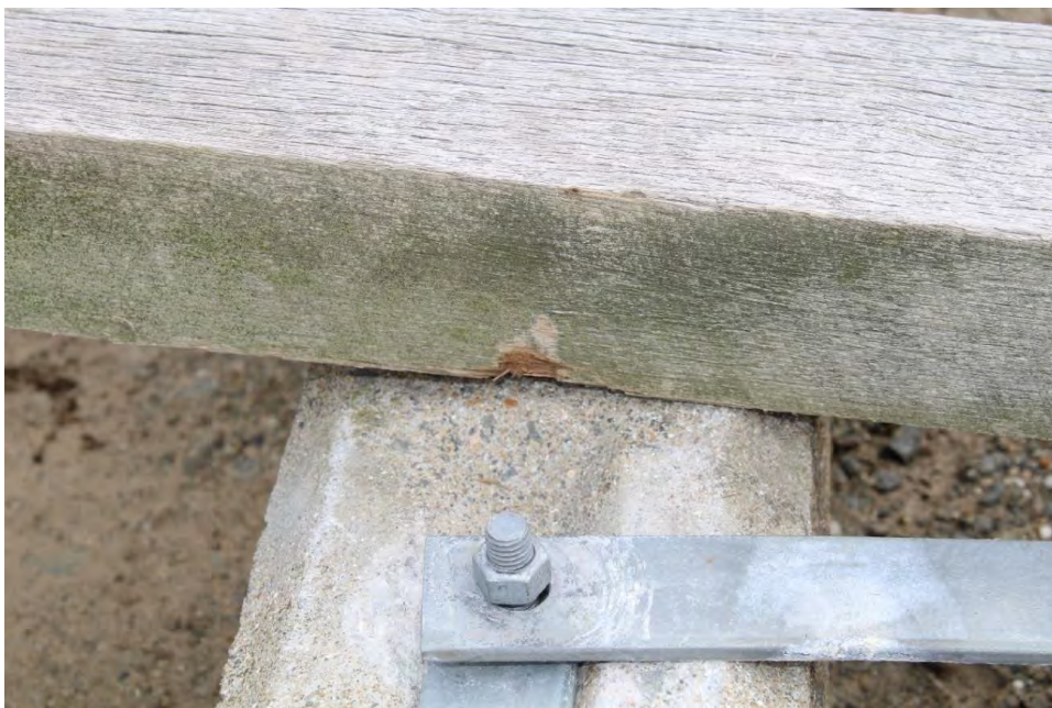
Fig. 61. Note fresh indentation in wooden cross-arm above bolt.
