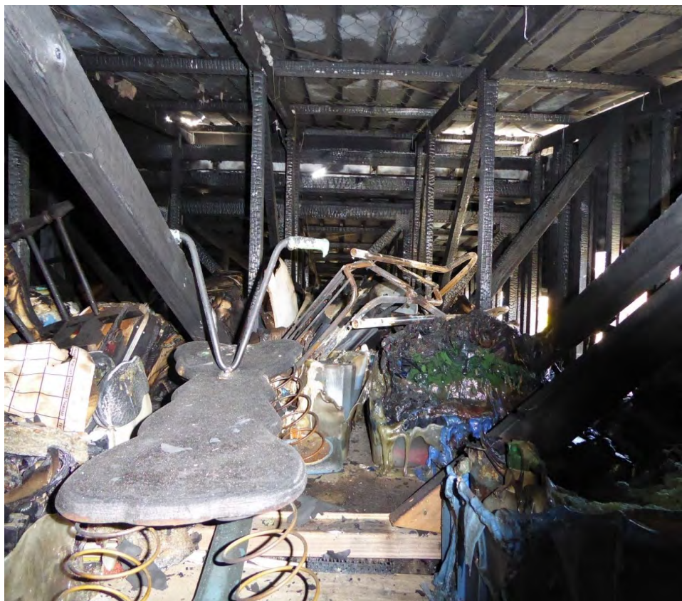
Fig. 18. A crew of firefighters entered this smoke-logged building, accessed the roof void by removing sections of ceiling in the lounge and kitchen and applied water into the roof space. This photo is taken in the roof space.
