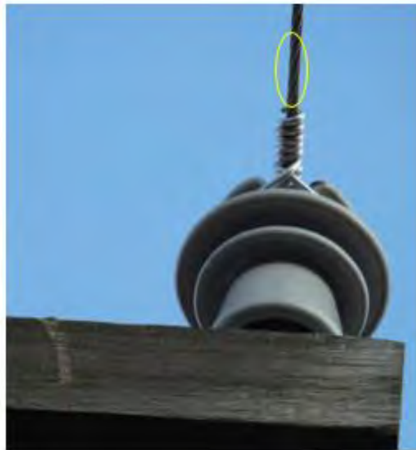
Fig. 51. Photograph above is a zoomed-out image of photograph (DSCF9362) the area within the yellow ellipse shows a rough edge that appears to be damaged.
