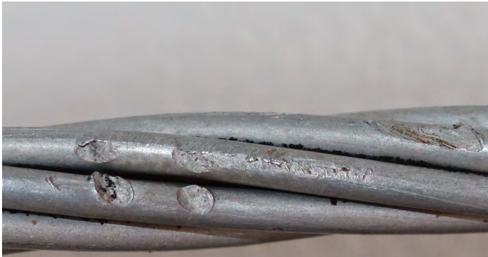
Fig. 83. Close up of arcing on twisted conductors IMG_1568.
