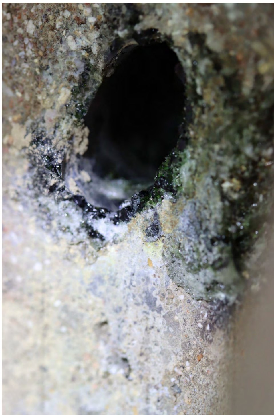
Fig. 72. Burn hole washer side of pole IMG_1452.
