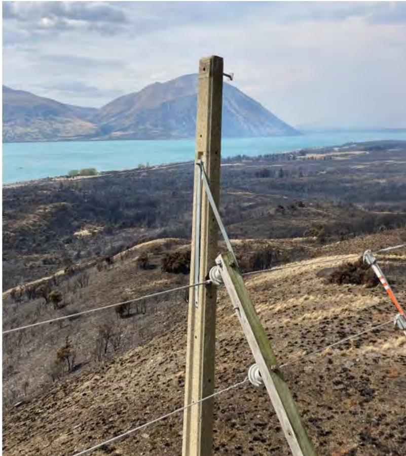
Fig. 80. Pole 35693 Blue Phase touching pole. (Photo supplied by Network Waitaki)
