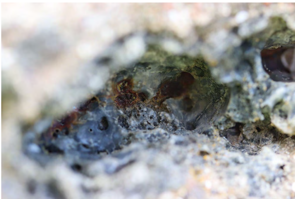
Fig. 79. Looking into old damage appears to display old heat damage. IMG_1485.JPG.
