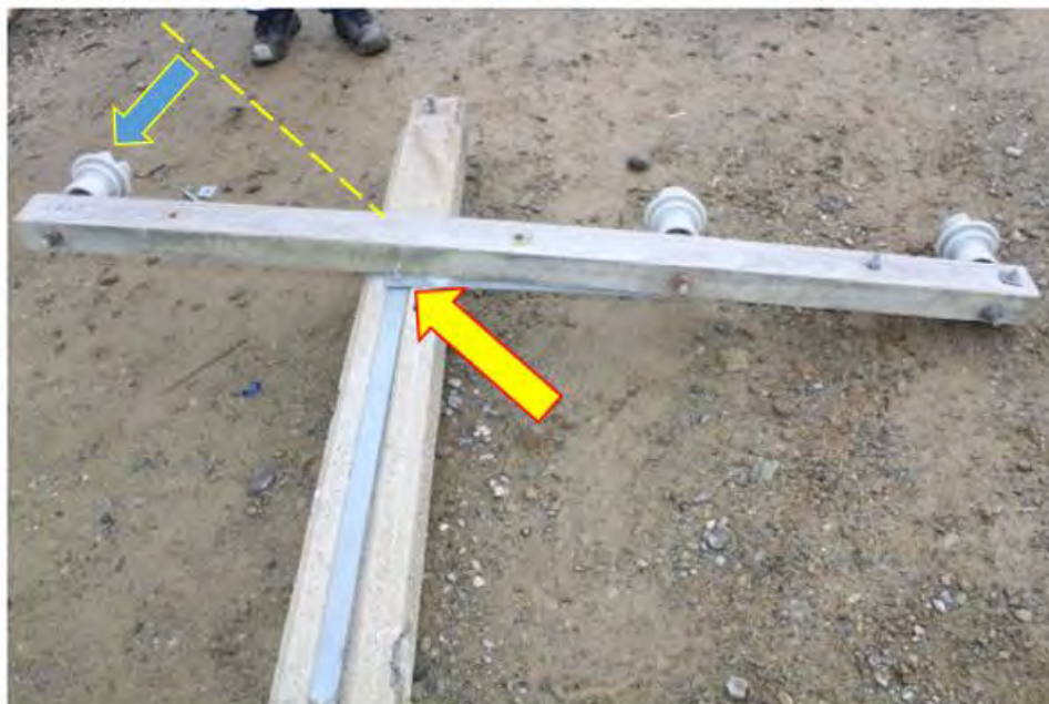
Fig.62. Above, position of metal lakeside stay arm above the RED phase. Held by tension on centre bolt.
