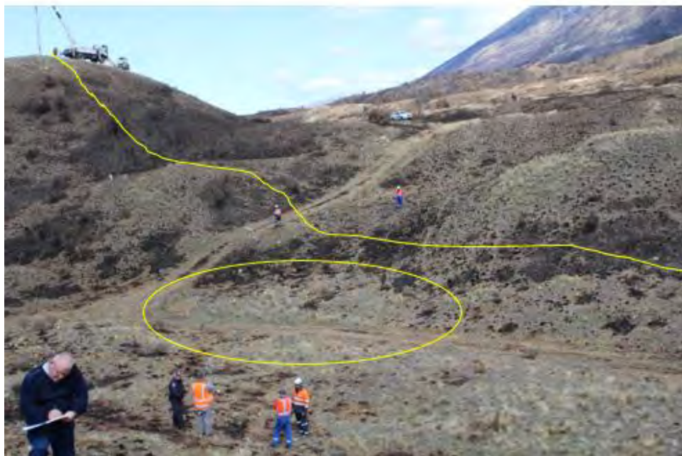
Fig. 39. Area of interest below damaged conductors between poles 870452 and 821215 Yellow line is identifying the conductors lowered to the ground. Yellow circle is the area of interest below the damaged conductors
