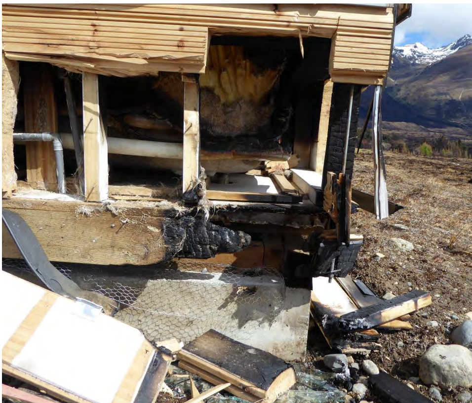
Fig. 20. An example of a partially damaged building due to ember transfer.
