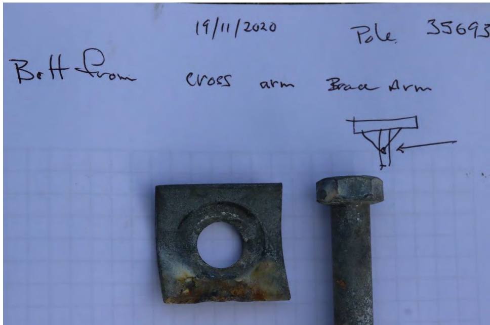
Fig. 76. Arc damage on bolt and washer – bolt holds both metal stay arms to centre of the pole. IMG_1444.JPG.
