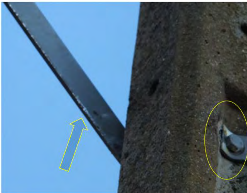
Fig. 49. Photograph (DSCF9369) above identifies location of damage to centre bolt, washer, and damage to edge of metal stay arm.
