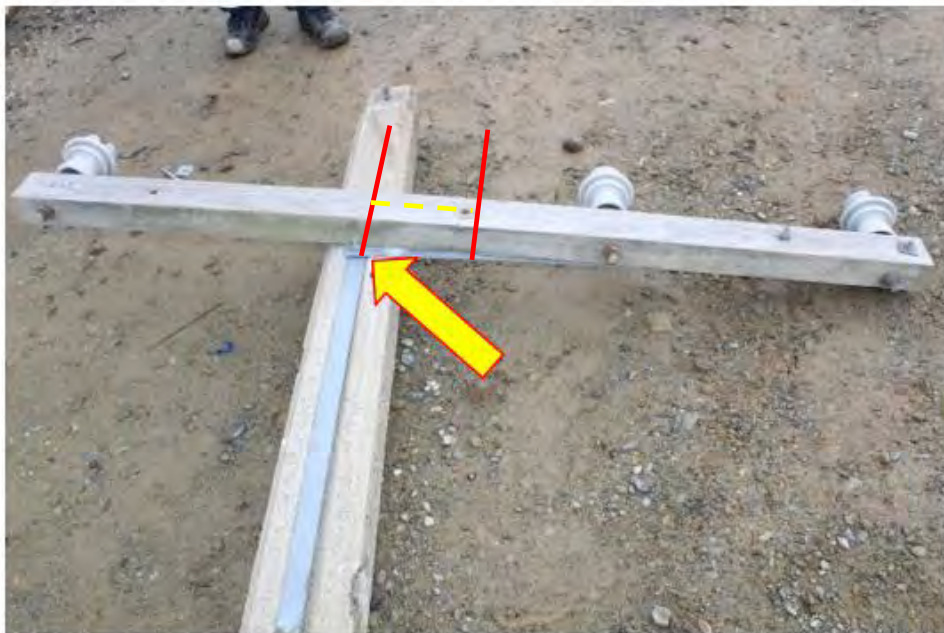
Fig. 59. Above, balancing position of wooden cross-arm after centre bolt vibrated backwards. Note: crossarm has displaced towards the hill side (right of pole) by approximately 250mm off centre.
