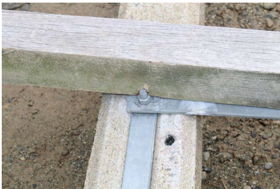
Fig. 60. Close up of cross-arm resting on bolt.
