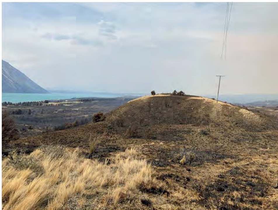
Fig. 40. Above shows lines that had have twisted but may not have made contacted each other. These lines are attached to pole 35693 spanning down to pole 17408 in the background.
