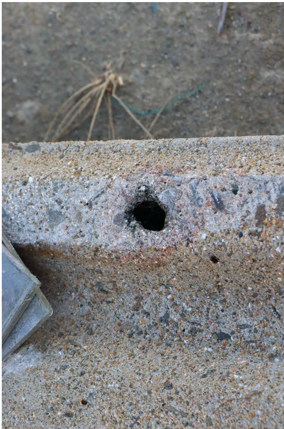
Fig. 65. Close up of the burn hole below the centre bolt holding the metal stay arms to the pole.
