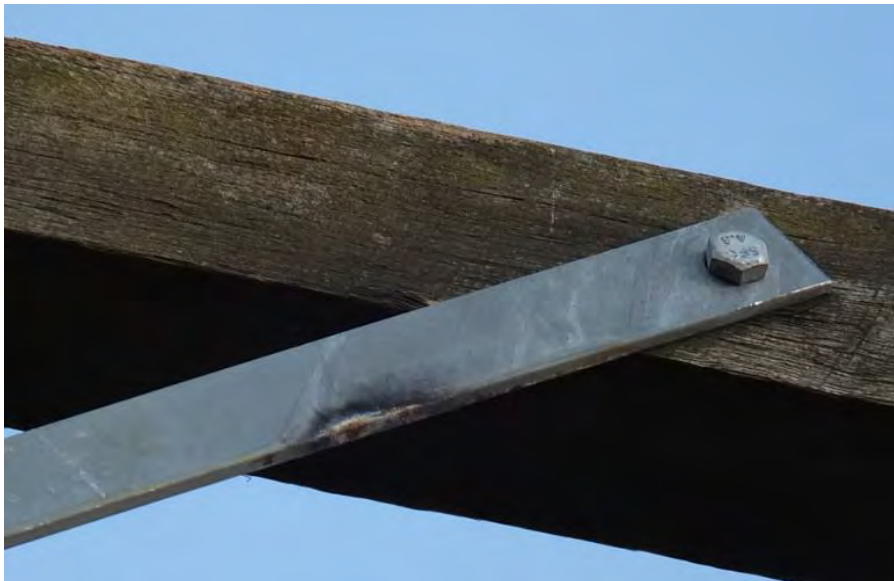
Fig.64. Arc mark of contact point on underside of Lakeside stay arm.
