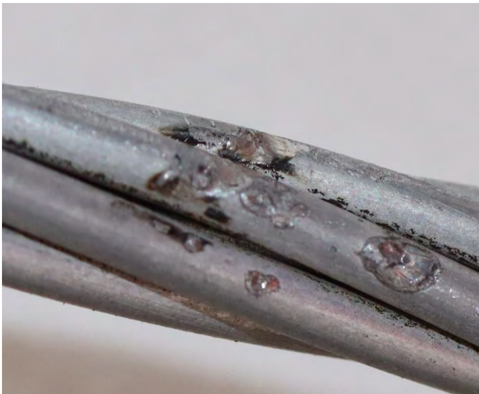
Fig. 84. Close up of arcing on twisted conductors IMG_1578.
