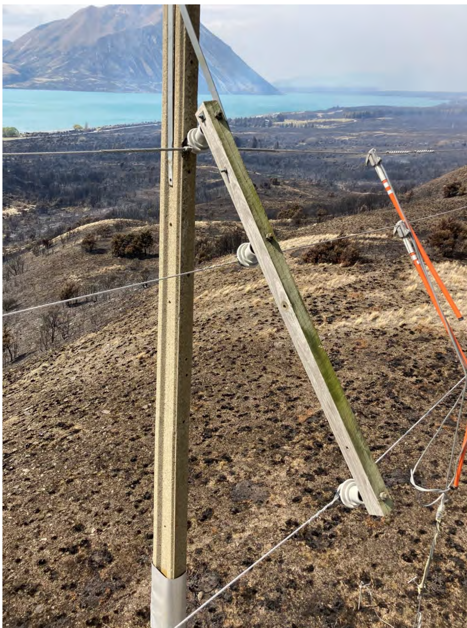
Fig. 55. Photograph (IMG_1711.JPG) above shows the cross-arm rotated over. Photograph supplied by Network Waitaki.
