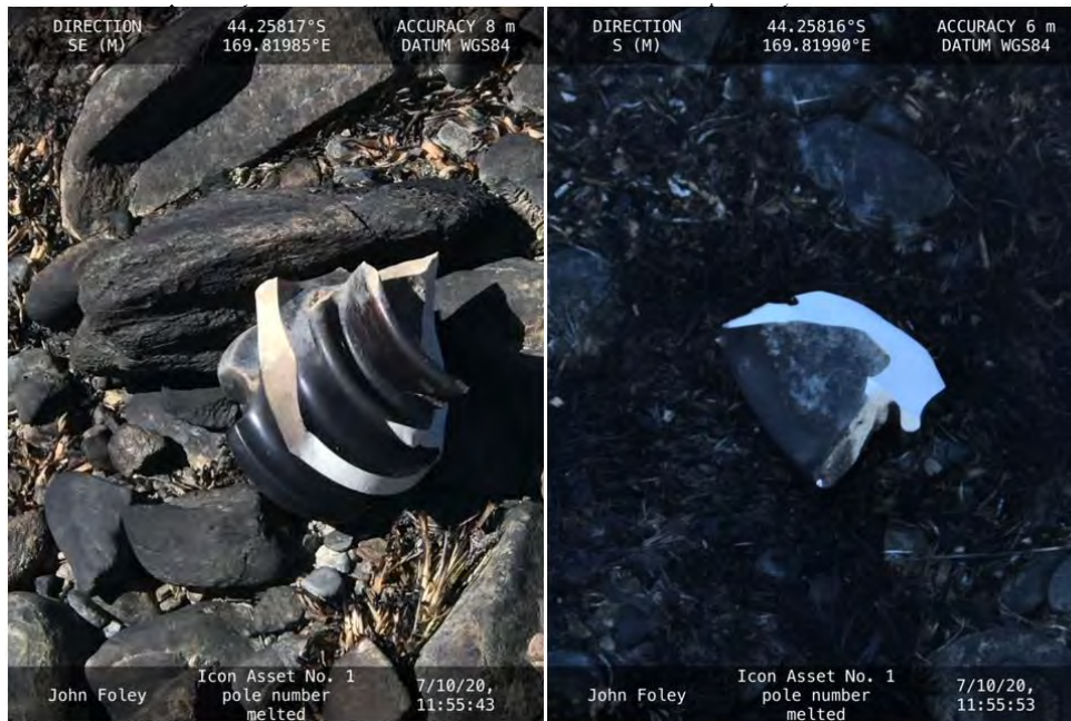
Fig. 41. and Fig. 42. Above, broken insulator located near pole.
