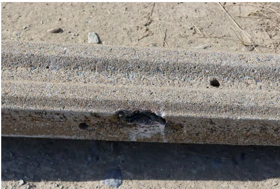
Fig. 78. Old damage on side of pole that lines up with the cross-arm when twisted over. IMG_1415.JPG.
