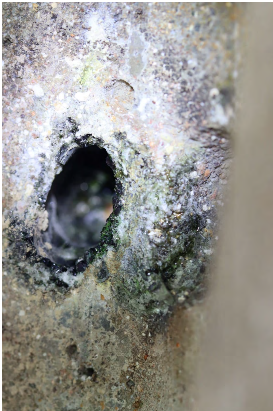
Fig. 71. IMG_1449.JPG edge of hole and surface of pole has been exposed to intense heat.
