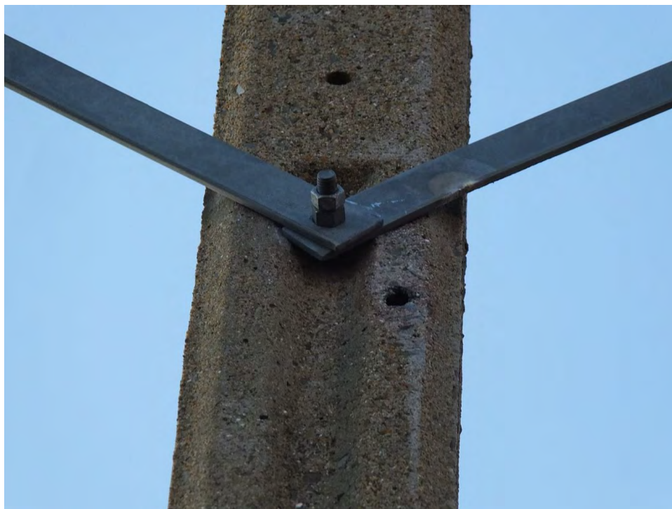
Fig. 48. Photograph (DSCF9365) above shows the lower arc mark on the hillside metal stay arm, a hole below the stay arm and what appears to be a scrape mark on the right-hand side of the pole below the metal stay arm.
