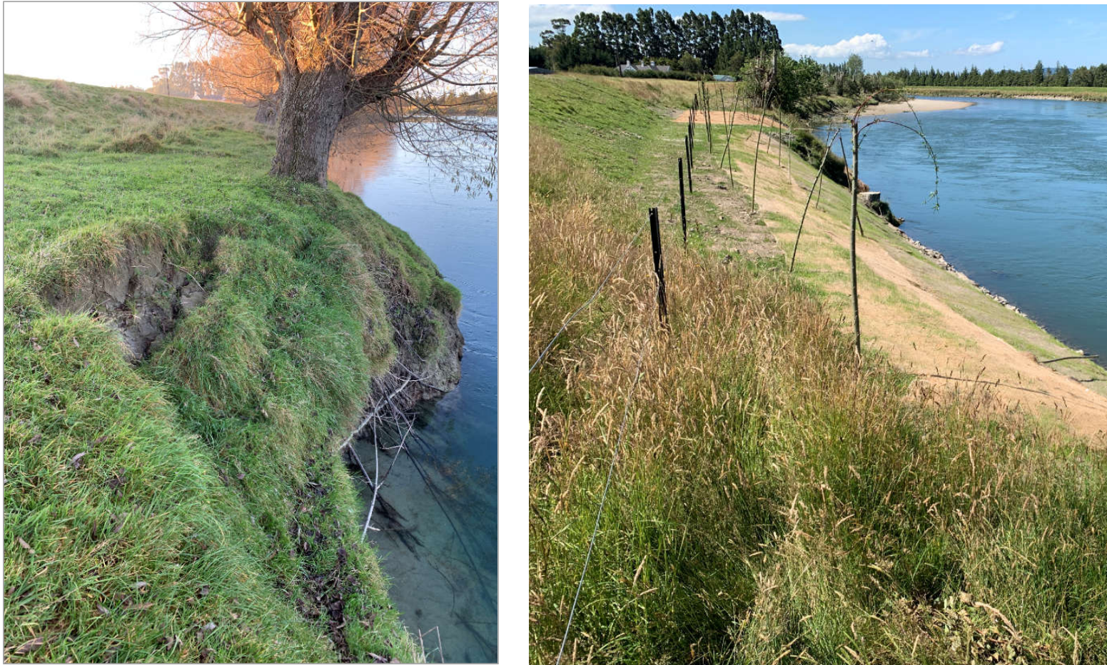
Figure 4. Riverbank Road floodbank at Lawsons (LC20), before(left) and after (right) reshaping and vegetation stabilisation.
