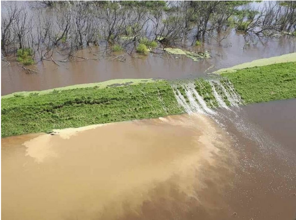
Figure 3. Waitepeka Floodbank showing slumping, overtopping and piping. 5 February 2020.
