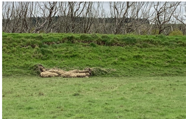
Figure 5. Slumping on floodbank (14 February 2020).
