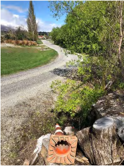
Figure 6 Butement Street on the land side of the Rees-Glenorchy Floodbank at the location assessed as vulnerable to damage instigated by scour.
