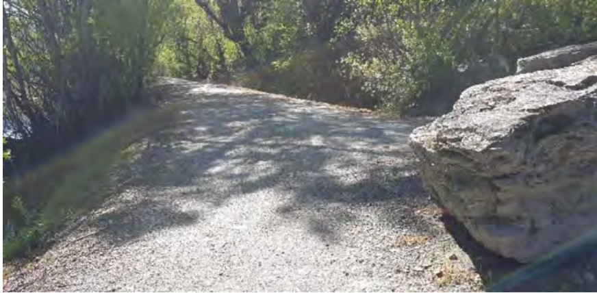
Figure 10 Embankment at location where culvert crosses under embankment. Potential area of interest for piping.
