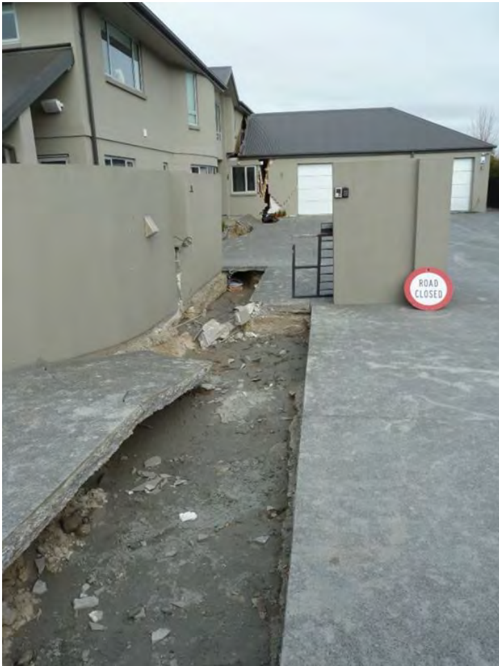
Figure B4 - Photo showing lateral spreading effects at Courtenay Drive, Kaiapoi following the 2010 Darfield earthquake. The ground crack filled up with liquefied sand and resulted in a significant evacuation hazard following the event. The lateral spreading at this site was approximately 2m.
