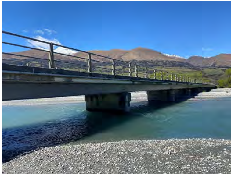
Close up photo of Rees River bridge further highlighting the limited capacity
