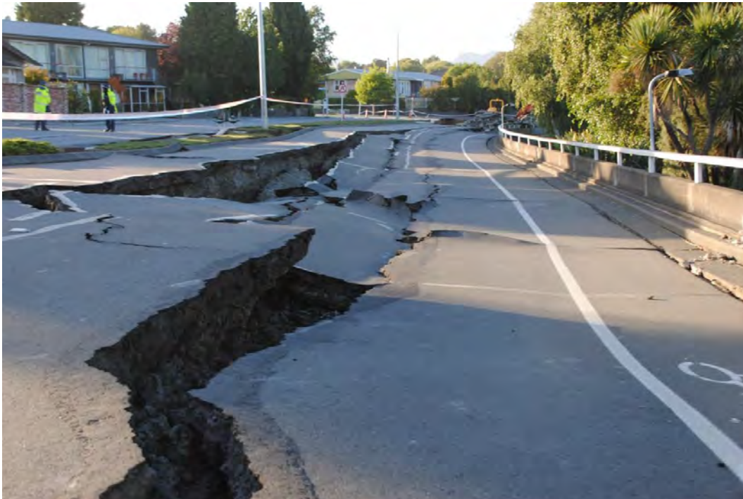
Figure B9 - Photo showing lateral spreading at Fitzgerald Ave, Christchurch following the 2011 Christchurch earthquake. The total lateral spreading at this site was approximately 2m. Vertical offsets in the order of 500mm (approx. 50% of the horizontal movement).
