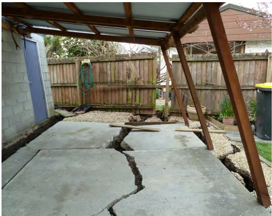
Figure B6 - Photo showing lateral spreading effects at Courtenay Drive, Kaiapoi following the 2010 Darfield earthquake. The total lateral spreading at this site was approximately 2m.
