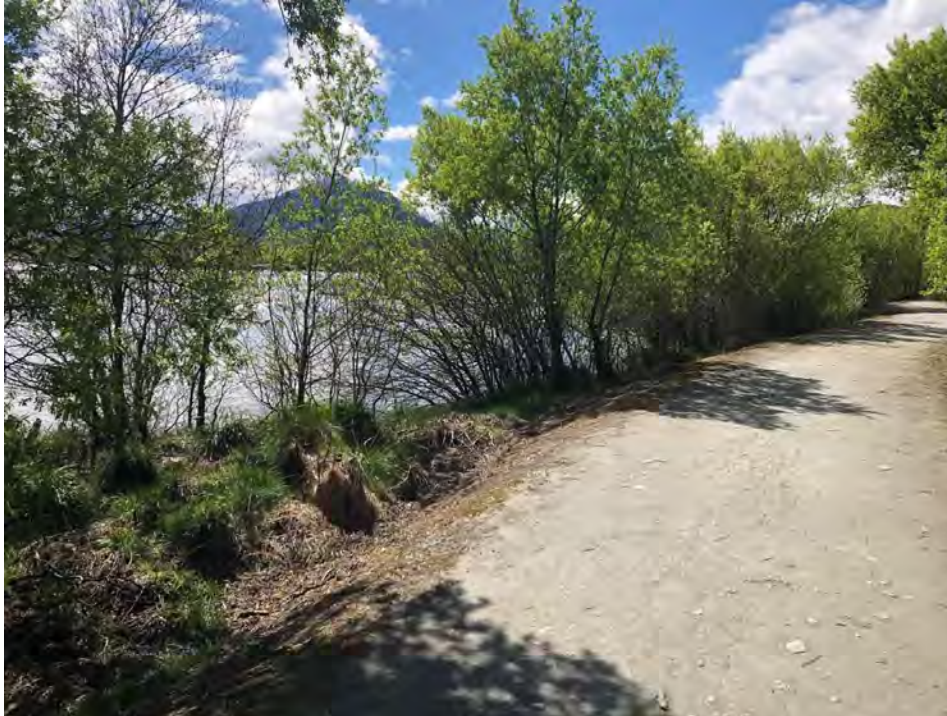
Figure 4 Rees-Glenorchy Floodbank adjacent to the Rees River confluence with Lagoon Stream. The Rees River is directed towards the Rees-Glenorchy Floodbank, increasing the likelihood of scour damage.
