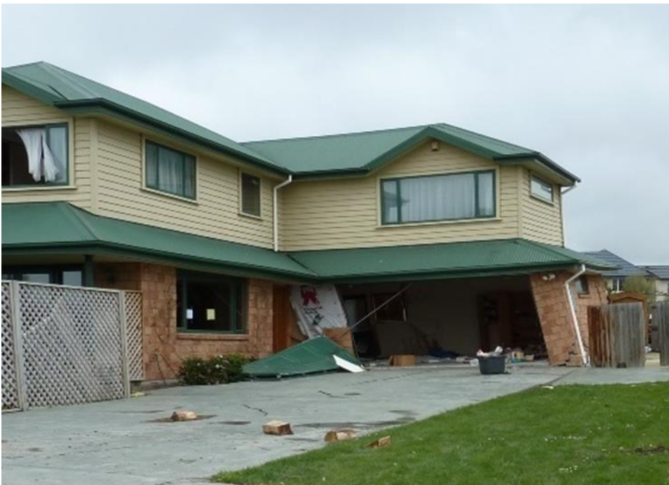
Figure B7 - Photo showing lateral spreading effects at Courtenay Drive, Kaiapoi following the 2010 Darfield earthquake. The total lateral spreading at this site was approximately 2m. If the lateral spreading at the site had been higher, this building would likely have collapsed.
