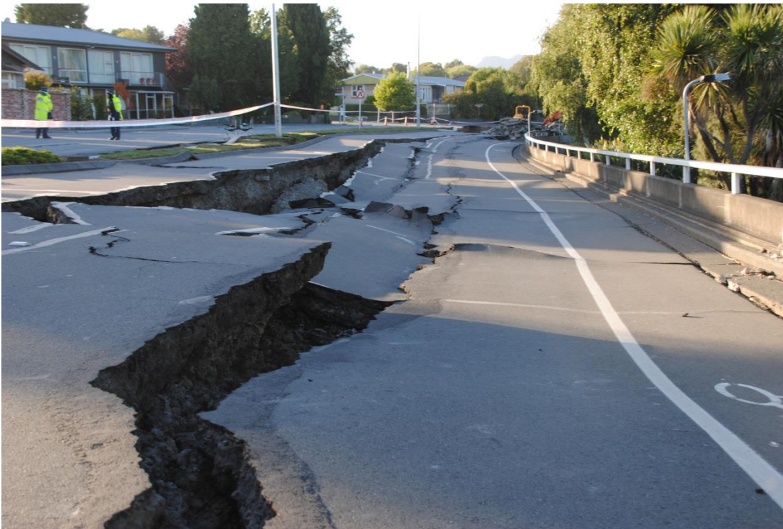
Figure B9 - Photo showing lateral spreading at Fitzgerald Ave, Christchurch following the 2011 Christchurch earthquake. The total lateral spreading at this site was approximately 2m. Vertical offsets in the order of 500mm (approx. 50% of the horizontal movement).
