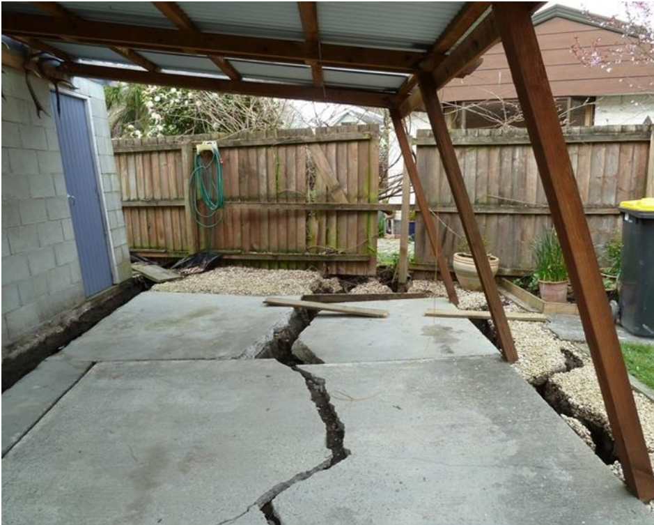
Figure B6 - Photo showing lateral spreading effects at Courtenay Drive, Kaiapoi following the 2010 Darfield earthquake. The total lateral spreading at this site was approximately 2m.
