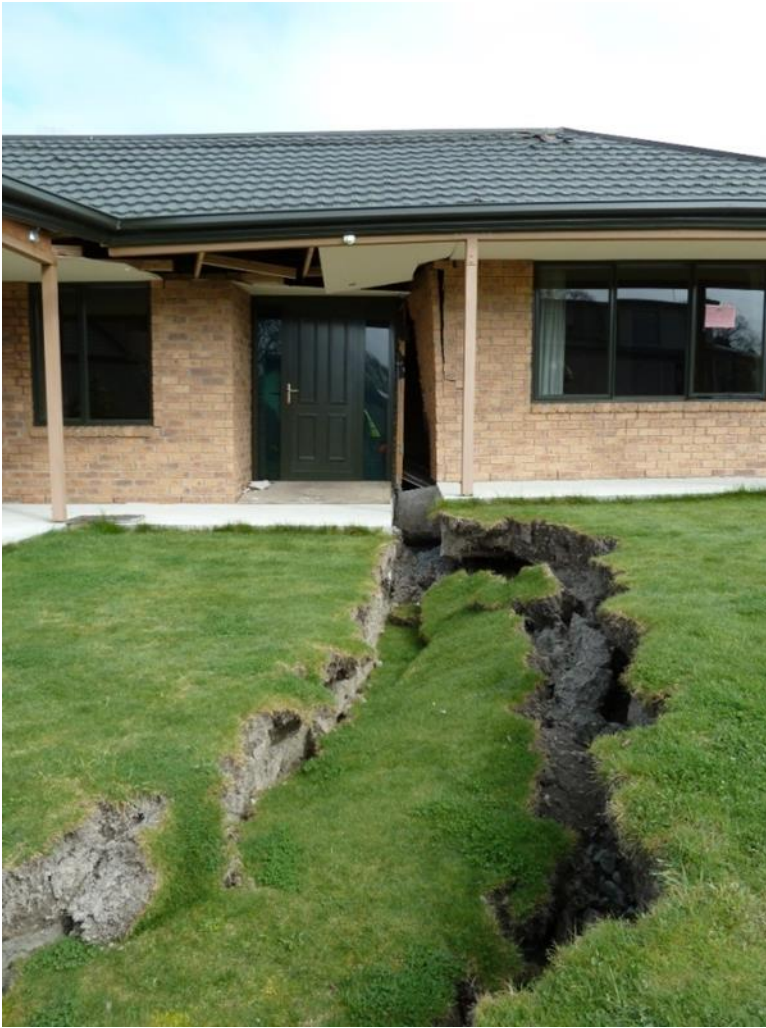
Figure B5 - Photo showing lateral spreading effects at Courtenay Drive, Kaiapoi following the 2010 Darfield earthquake. The lateral spreading caused approximately 1m of horizontal stretch and also a 300mm vertical offset. The total lateral spreading at this site was approximately 2m.
