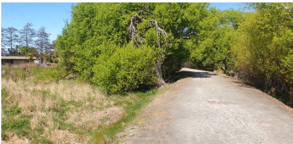
Figure 9 Embankment at location inferred by WSP to be an area of interest for possible piping.
