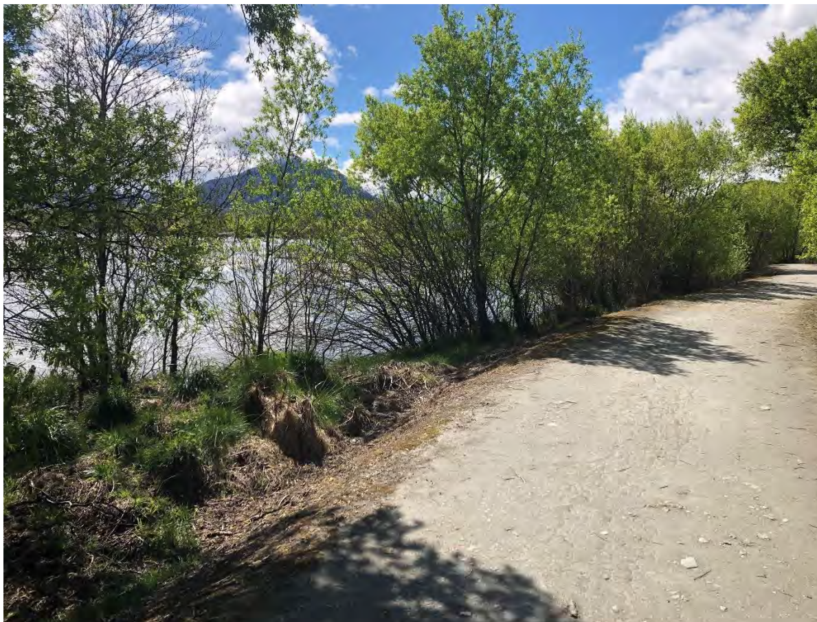
Figure 4 Rees-Glenorchy Floodbank adjacent to the Rees River confluence with Lagoon Stream. The Rees River is directed towards the Rees-Glenorchy Floodbank, increasing the likelihood of scour damage.
