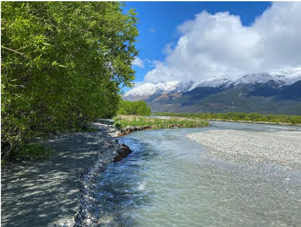
Photo of erosion on left bank of the Rees River (Rees Valley Station) – this photo also highlights the lack of available freeboard for the Rees River before it overflows onto the left bank
