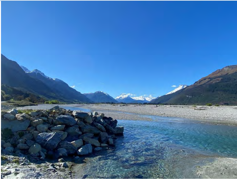
Example of a typical rock groyne constructed on the true right bank of the Dart River with significant scour on the downstream side of the groyne.
