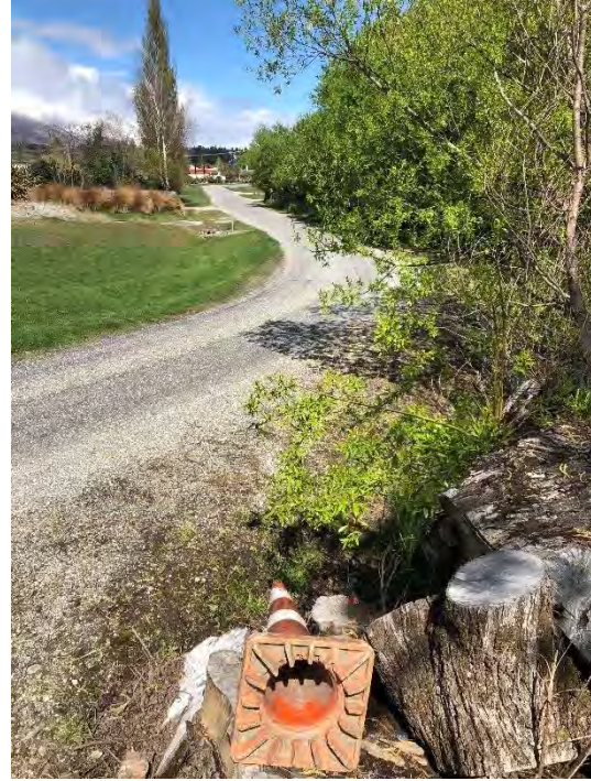
Figure 6 Butement Street on the land side of the Rees-Glenorchy Floodbank at the location assessed as vulnerable to damage instigated by scour.
