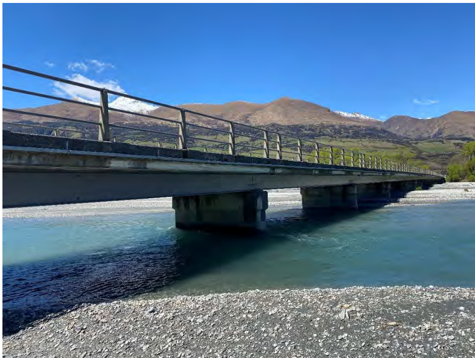
Close up photo of Rees River bridge further highlighting the limited capacity
