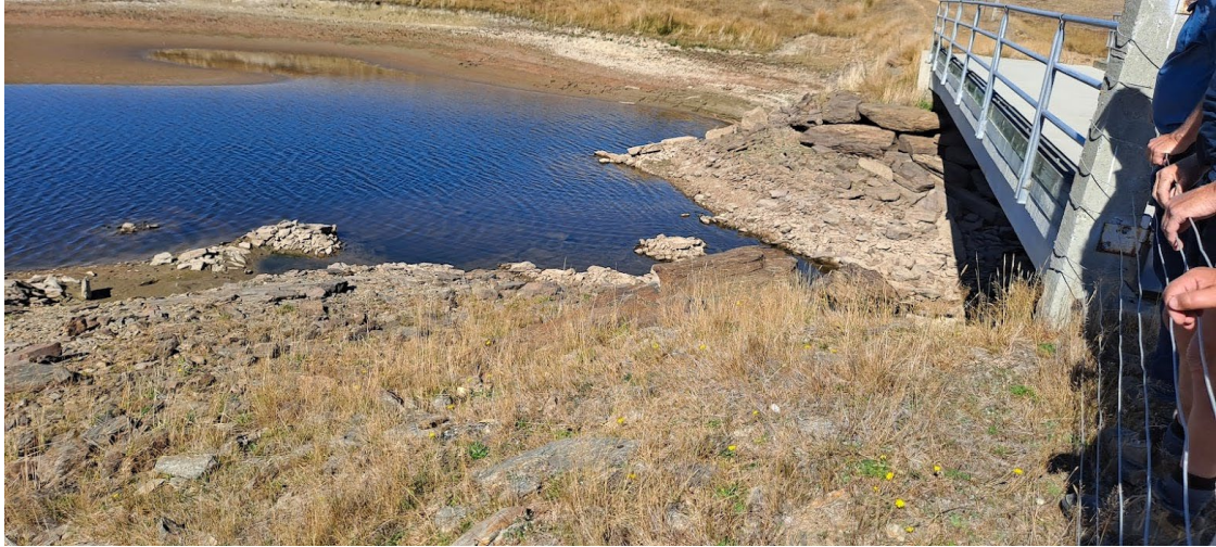
Photo 17: Weir under causeway at north branch that holds water levels up as lake level drops
