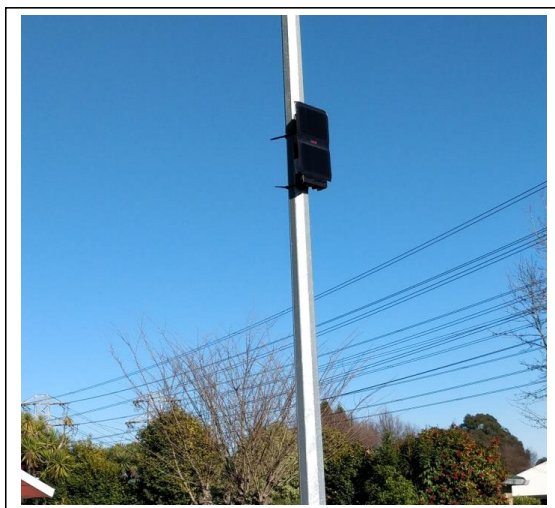
Figure 1: A typical ODIN installation on a roadside light pole.
