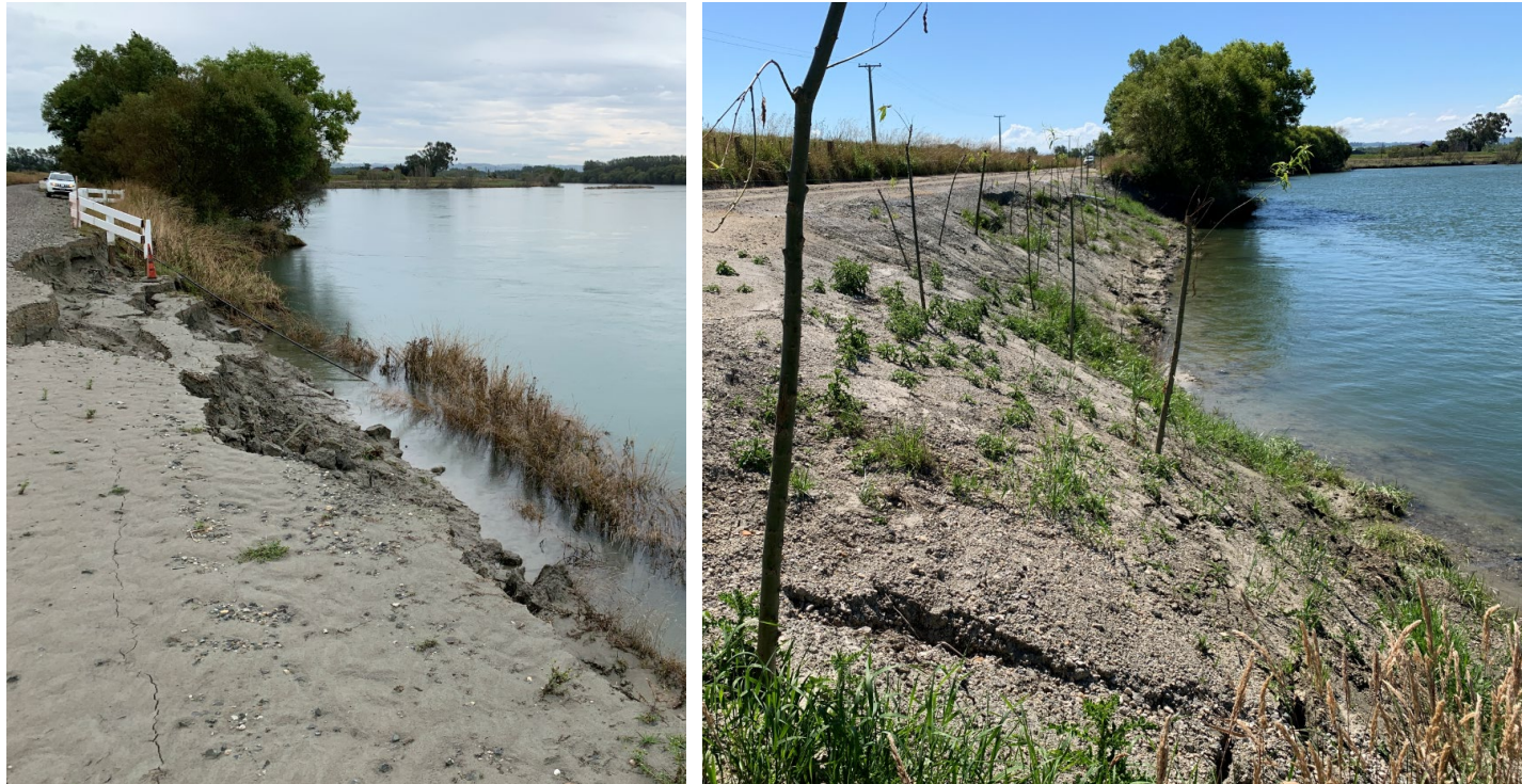
Figure 2. Riverbank Road at Renton Road (LC17) floodbank before and after reshaping and vegetation stabilisation.
