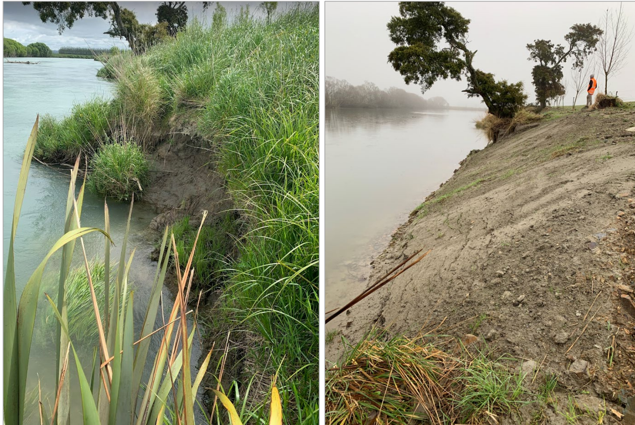
Figure 7. Floodbank stabilisation at 625 Riverbank Road (LC14), before (left) and after (right) bank stabilisation and revegetation reinstatement. One of 10 repairs at this site.
