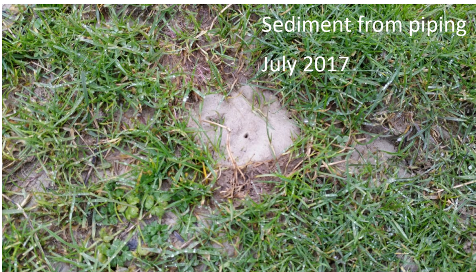
Figure 4. Areas where piping was observed in 2017 and sedimentation from piping.
