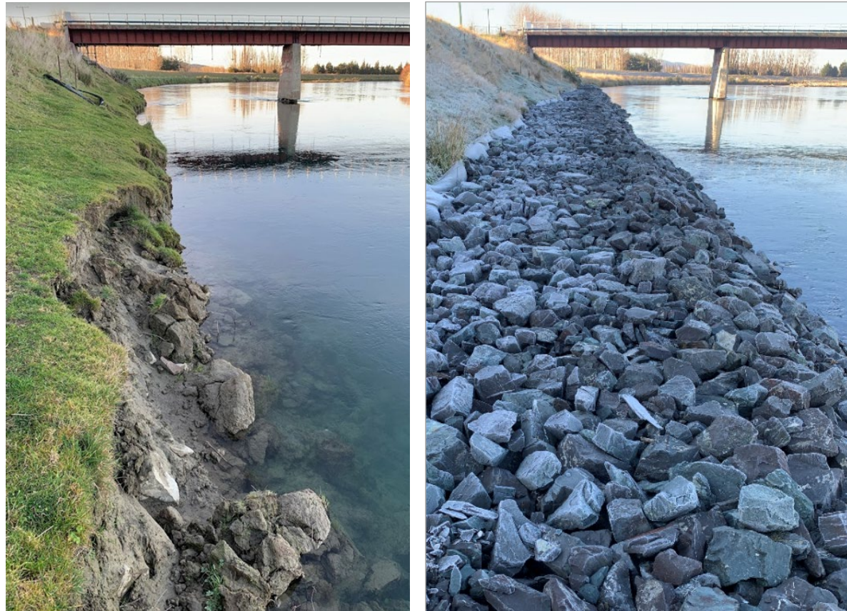
Figure 5. Riverbank Road floodbank at bridge near Stirling (LC21), before(left) and after (right) reshaping and vegetation stabilisation.
