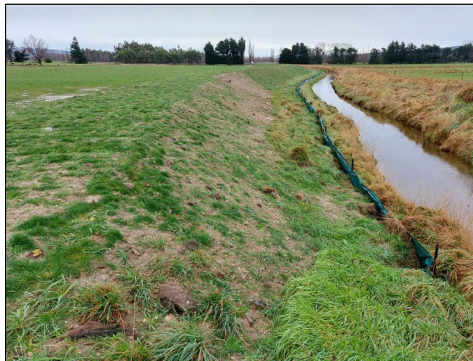
Figure 4. Stage 5 complete. Silt fence to be removed once grass seeding has fully established itself.
