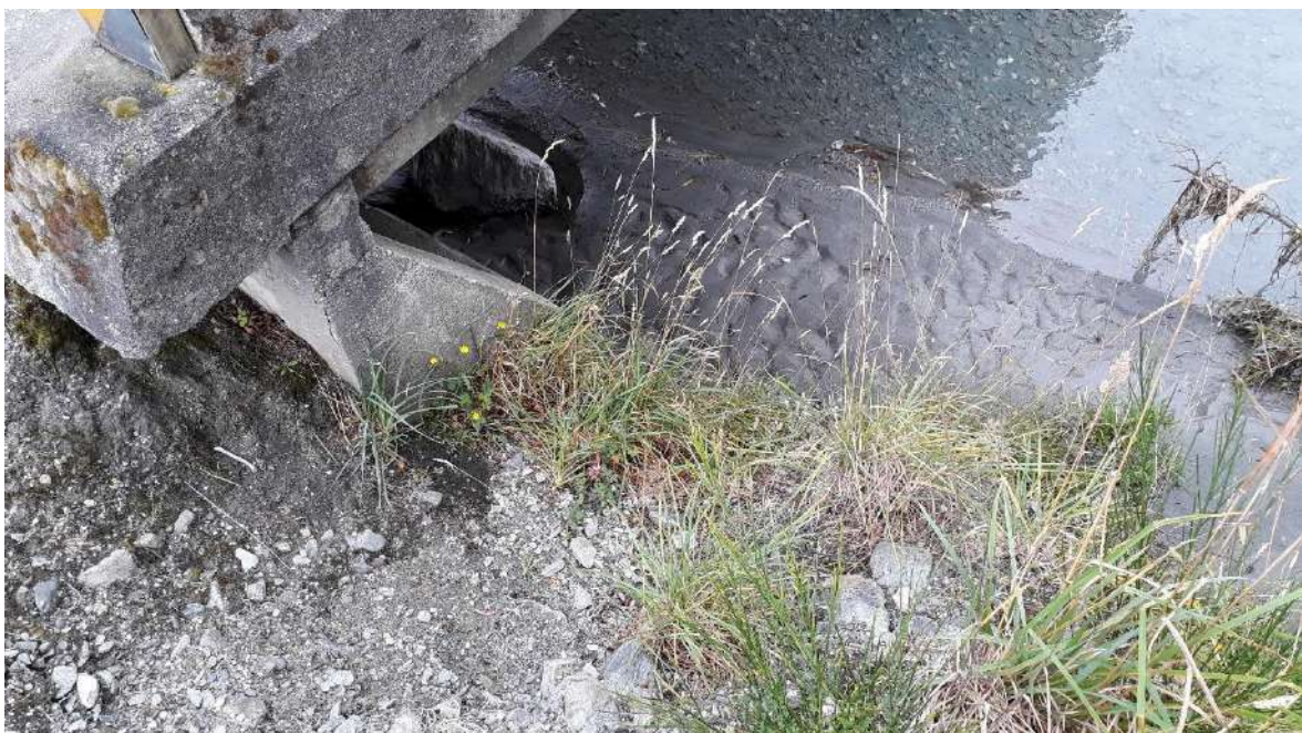
Figure 6.2: View under left abutment of Rees Bridge from upstream side of road embankment showing small amount of slumping of approach embankment fill material
