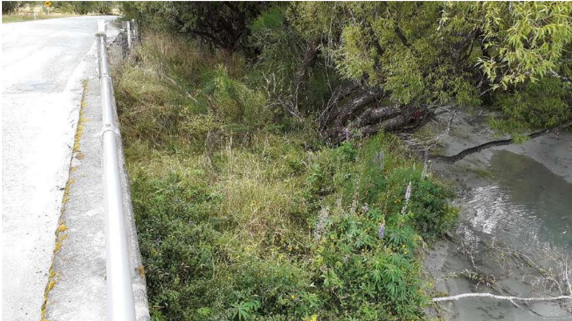
Figure 6.3: View of right abutment of Rees Bridge on upstream side from bridge
