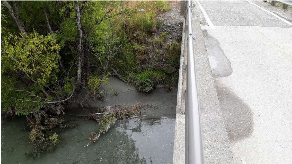
Figure 6.1: View of left abutment of Rees Bridge on upstream side from bridge
