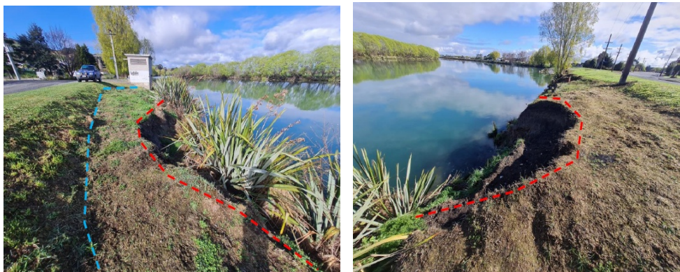
Photos 2 (L) and 3 (R) showing the vulnerability of an erosion site at Lower Clutha at the Kaitangata site location of the Lower Clutha Flood Protection Scheme.
