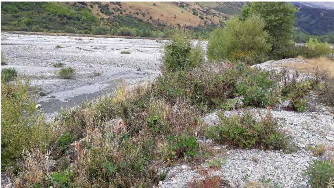
Figure 6.7: Rock groyne structure on right bank of Rees River upstream of existing bridge (the head of the structure beyond the willow saplings in the right of the photo was damaged in a recent flood event)
