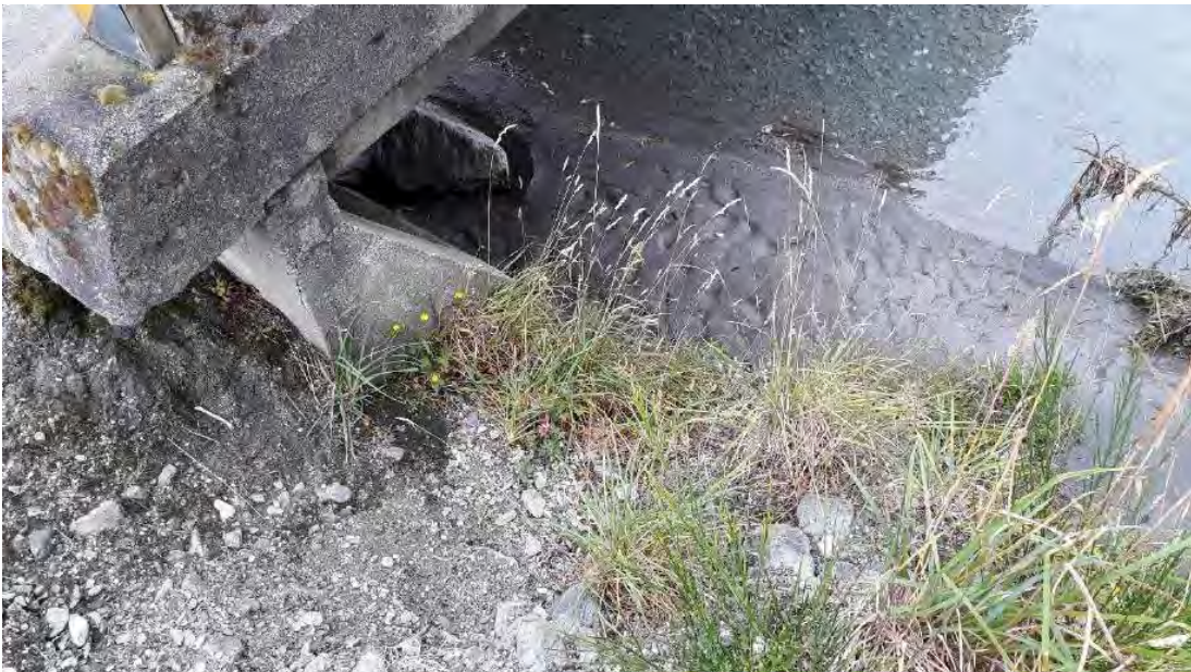
Figure 6.2: View under left abutment of Rees Bridge from upstream side of road embankment showing small amount of slumping of approach embankment fill material
