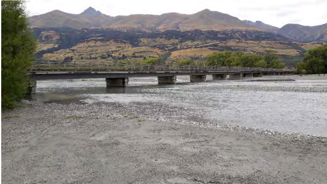
Figure 2.6: Riverbed aggradation under Rees Bridge in February 2022 (viewed looking upstream)
