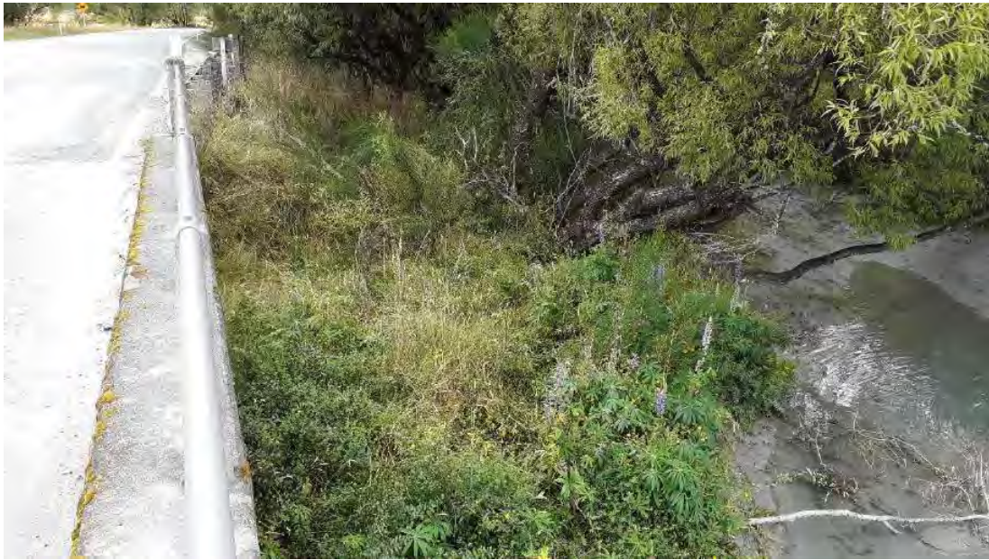
Figure 6.3: View of right abutment of Rees Bridge on upstream side from bridge
