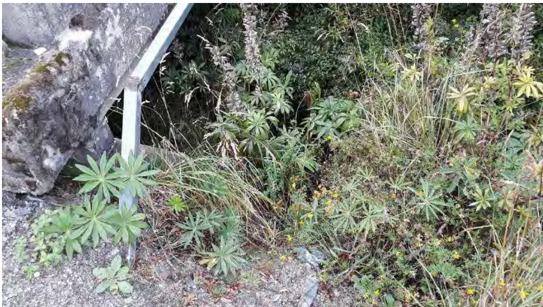
Figure 6.4: View under right abutment of Rees Bridge from downstream side of road embankment
