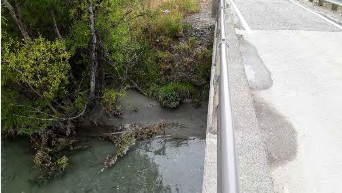
Figure 6.1: View of left abutment of Rees Bridge on upstream side from bridge
