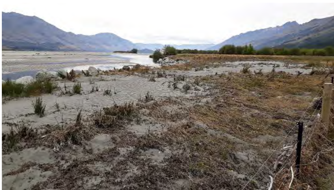
Figure 2.5: Erosion protection works adjacent to Kinloch Road with evidence of recent breakout flows across road in February 2022 (note level of riverbed adjacent to right bank floodplain)
