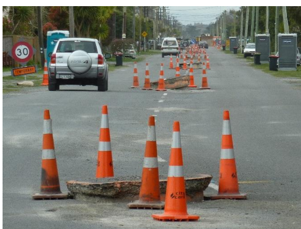
Stormwater manholes that have floated up out of the liquefied ground.
