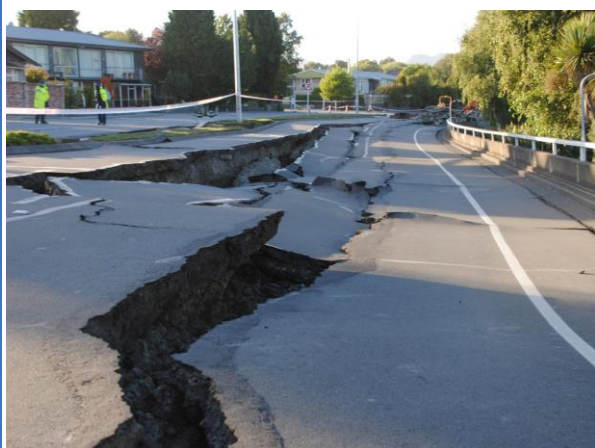
Lateral spreading caused a series of 0.5m cracks and drops in this road.
