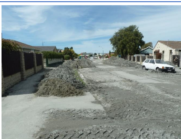
Liquefied sand on the street, with piles of sand shovelled out from under and around houses.
