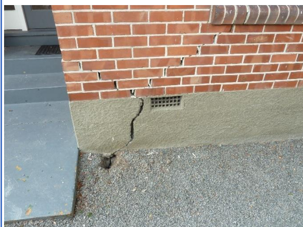
Foundation and brickwork damage.
