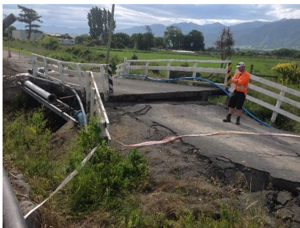
Lateral spreading buckled this bridge and damaged the approaches, cutting the main trunk water supply and fibre optic cable running across the bridge.
