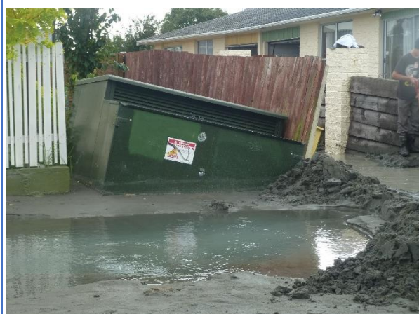
Power transformer that has sunk into the liquefied ground.
