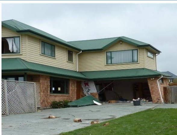
A 1m wide ground crack ran through the middle of this house, pulling the garage walls apart.
