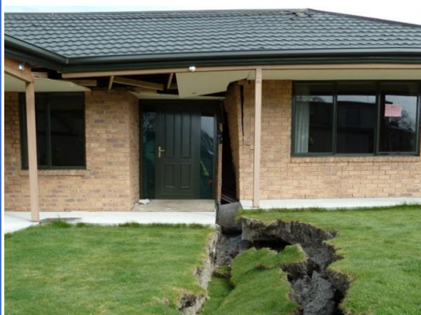
The cracks running under this house caused the front part to pull away and drop 0.5m.
