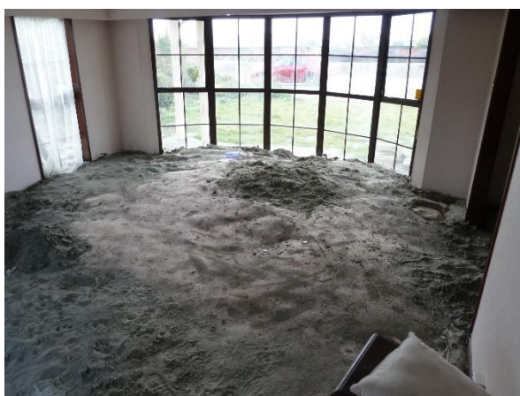
Liquefied sand that has broken through the floor slab and filled up inside the house.
