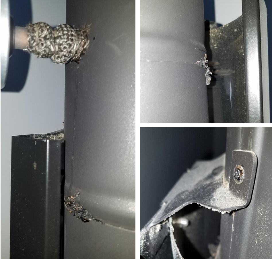
Figure 21 Household 1 Flue Showing Build-up of Creosote
