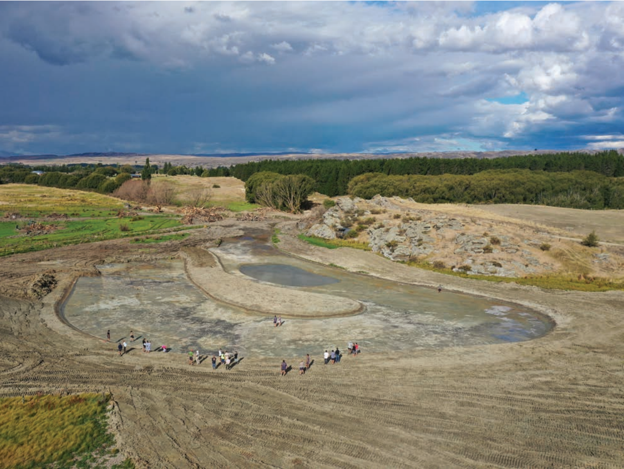
Image 6: A catchment fieldday held on 3 March 2023 in the partly constructed wetland, which is an important part of the farmer-led Thomsons Catchment Project in the Manuherehia Catchment to improve water quality. Source: Thomsons Catchment Project
