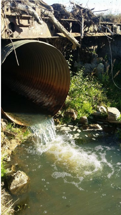
Figure 10. Track culvert in Watkins Creek perched above the stream. No passage upstream can occur as the overhanging lip would prevent even most climbing species.
