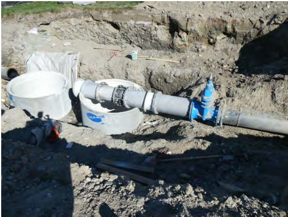
Figure 6: Mill Creek (Arrow River water) augmentation works under construction, manholes and pipework.
