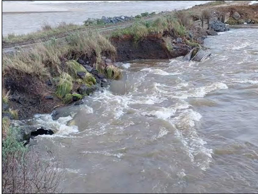
Figure 9: Erosion damages to the southern (Puerua River) side of the Koau mouth training line structure (June 2023).
