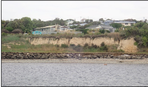
Kakanui Estuary margin, artificial rock walls in the lower and mid estuary (top) and natural steep banks (bottom)
