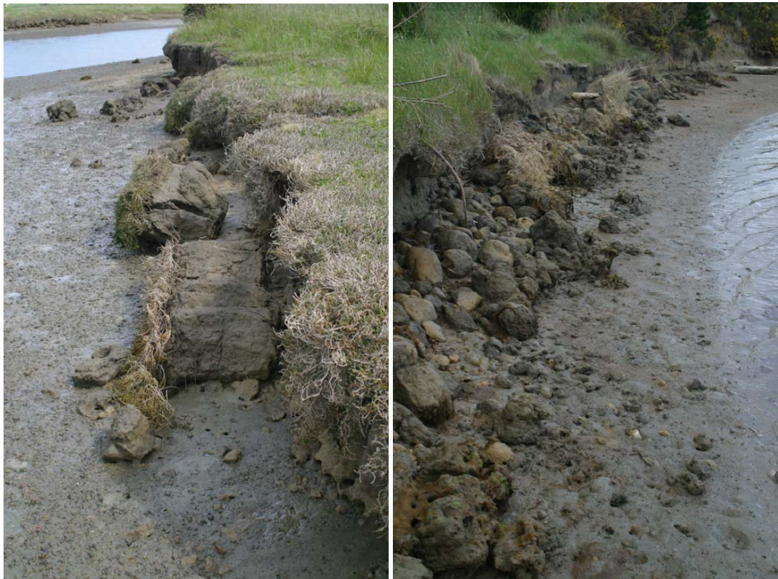
Figure 2. Evidence of relatively recent erosion along two of the main water channels, Shag River Estuary.
