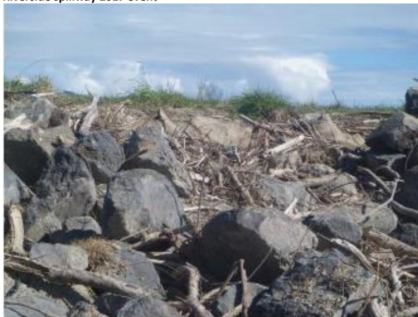
Photo 8: Image showing crest damage to Riverside Spillway, July 2017.
