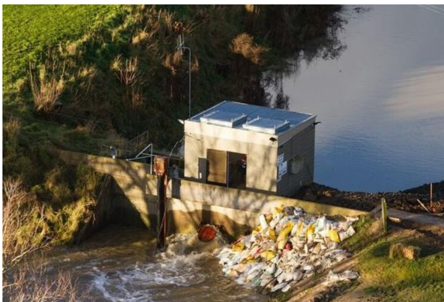
Photo 4: Image showing Mill Creek Pump Station after 2017 July event.
