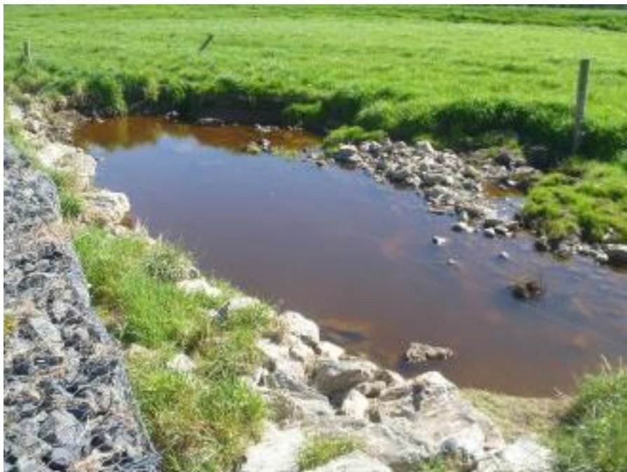
Image 9: Scour damage downstream of Riverside spillway gated section, July 2017
