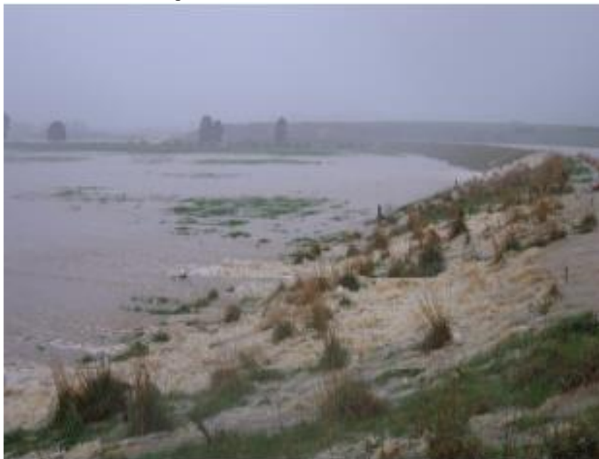
Photo 5: Image showing Contour Channel overtopping downstream of Otakia Road, April 2006.
