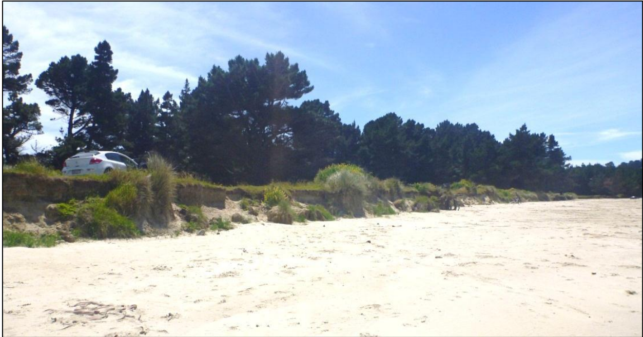
Figure 68 Evidence of recent erosion of Holocene beach deposits at the north-eastern end of Waikouaiti Beach, alongside Matanaka Drive (December 2013)
