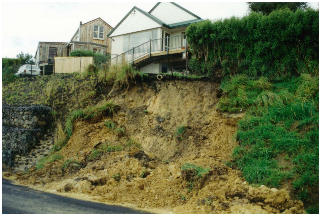
Figure 11 A small surficial landslide from this road cut in Margate Ave, Broad Bay, resulted from the March 1994 rainstorm. Flow from the drain at the head of the slide may have contributed to the failure. However, the gabion wall to the left indicates that this slope has previously experienced instability, which the gabions were doubtless installed to remediate. This photo illustrates the potential hazard of landslide movement undermining a property. Photo: GNS Science, I.M. Turnbull, 20 March 1994.
