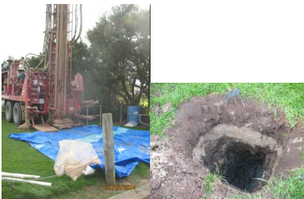
Photograph 2 Drilling rig at Culling Park, Photograph 3 Hand dug pit prior to drilling of bore
