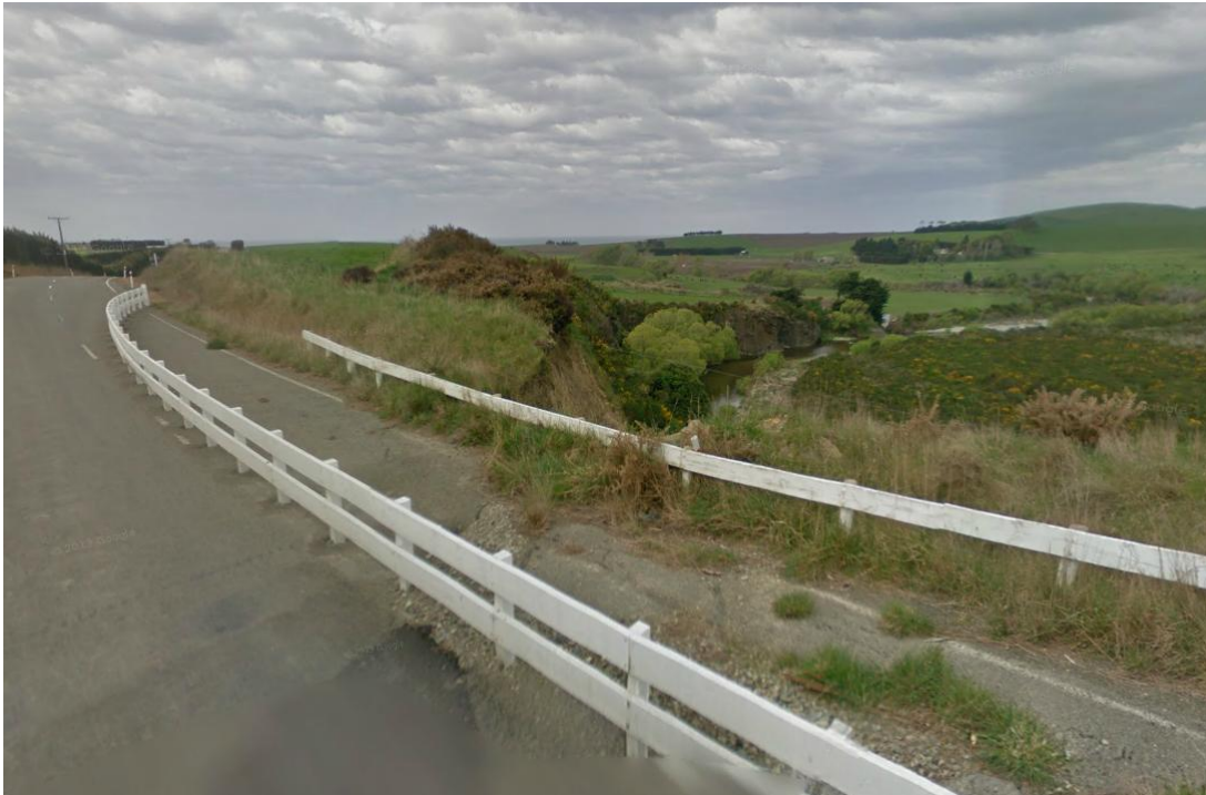
Figure 6-Section of bank erosion on the true left of the Waianakarua River below Waianakarua Road (Google Maps, Street view) (October 2012)
