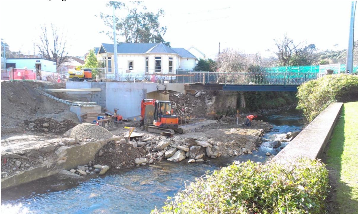
Photograph 1 – Modifications to the St David Street footbridge. The new foundation beam for the supporting pier can be seen to the right of the excavator.
