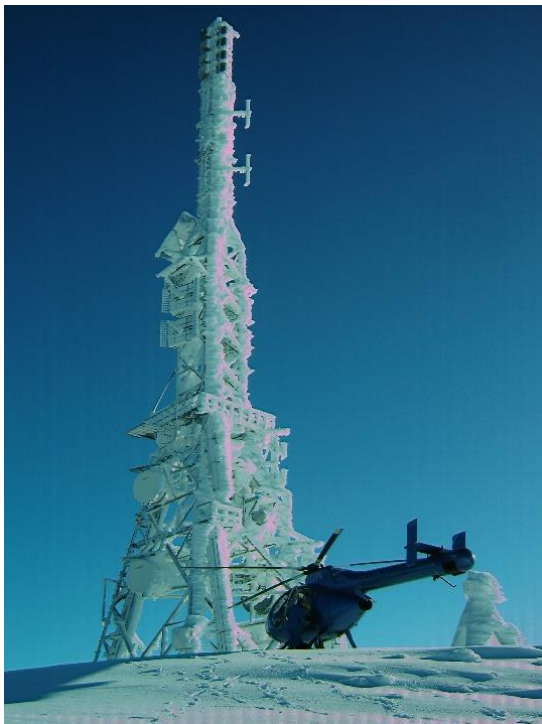
Helicopter Access to Transmission Site
