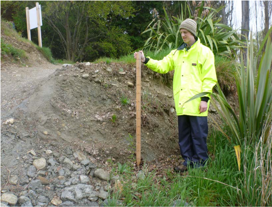
Figure 6. Perimeter scarp of the upstream landslide, which produces an abrupt step in the QLDC cycle track (October 2014).
