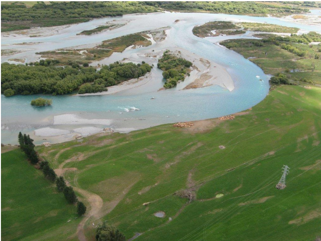
Photograph 10. Groynes being constructed on Irving property, true-left bank (56.4km) to reduce erosion risk for Transpower pylons.
