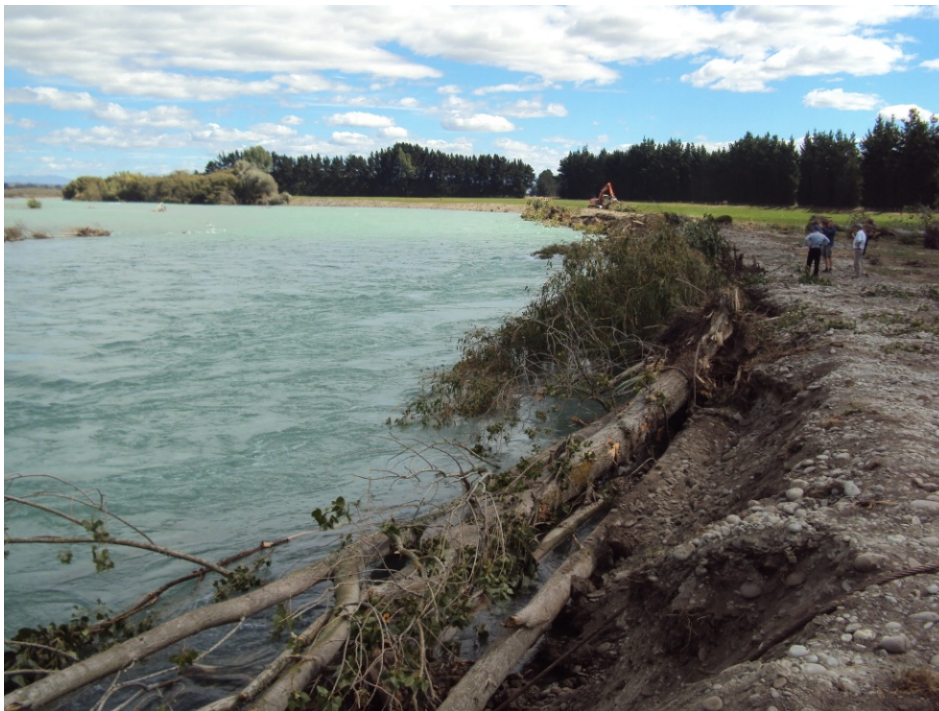
(a) Figure 1. Anchored tree protection being constructed on north bank on 4 March 2013 (a) in response to bank erosion observed 5 February 2013
