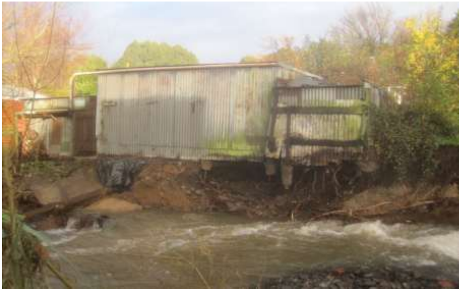
Figure 28. Bank erosion undermining a shed alongside Lindsay Creek at Kelvin Road, 4 June 2015
