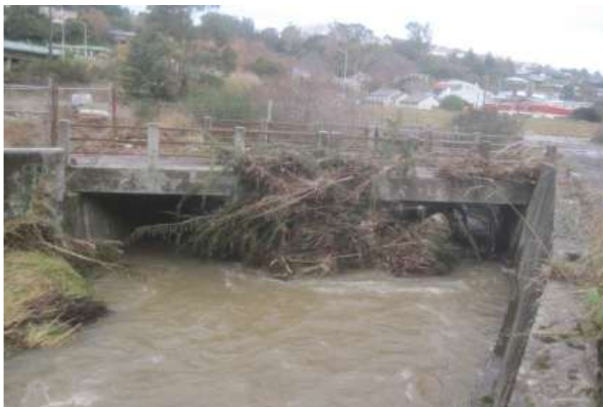
Figure 34. Tree and debris trapped under bridge at Burnside, 3 June 2015
