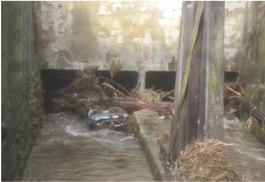
Figure 33. Car and tree lodged in culvert beneath SH1 at Burnside, 3 June 2015
