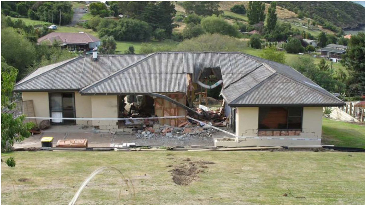
Figure 8. Rockfall damage to dwelling at Rapaki, Christchurch, during Feb 22nd 2011 earthquake. The gouge in the foreground is an impact divot from a boulder, which then impacted the house (Photo courtesy D. Barrell, GNS Science).
