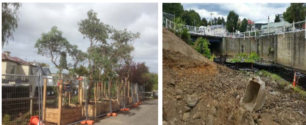
Figure 1 Dundas Street to St. David Street Reach of the Water of Leith showing Relocated Rhododendrons and Bulk Earthworks
