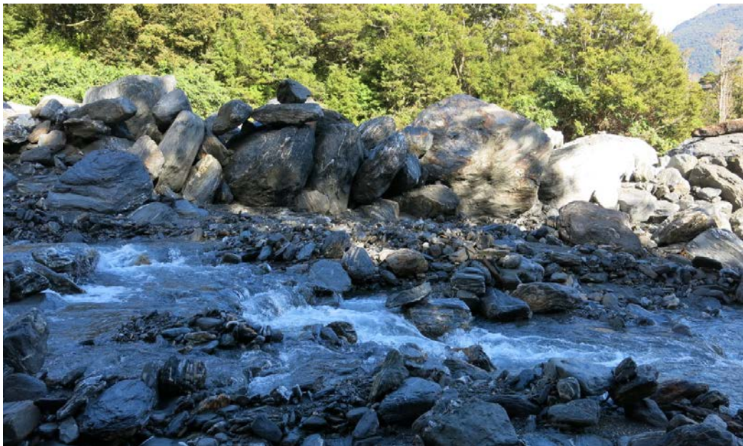
Figure 3: The Makarora River channel had changed markedly since the last inspection in April 2015 and there was evidence the flow had escaped the channel in many locations on the mid-to-lower fan surface. Pictured are a newly emplaced train of imbricated boulders, the largest measuring 3-4 m across. Note the rocks and log resting on top of the boulders.
