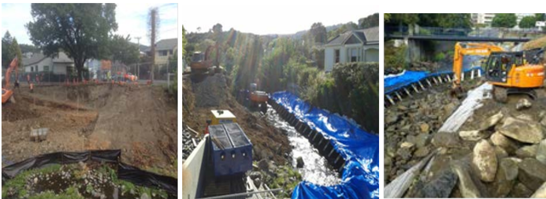
Figure 5: Dundas Street to St. David Street Reach of the Water of Leith showing cofferdam, placement of rock riprap, and completed bulk earthworks.
