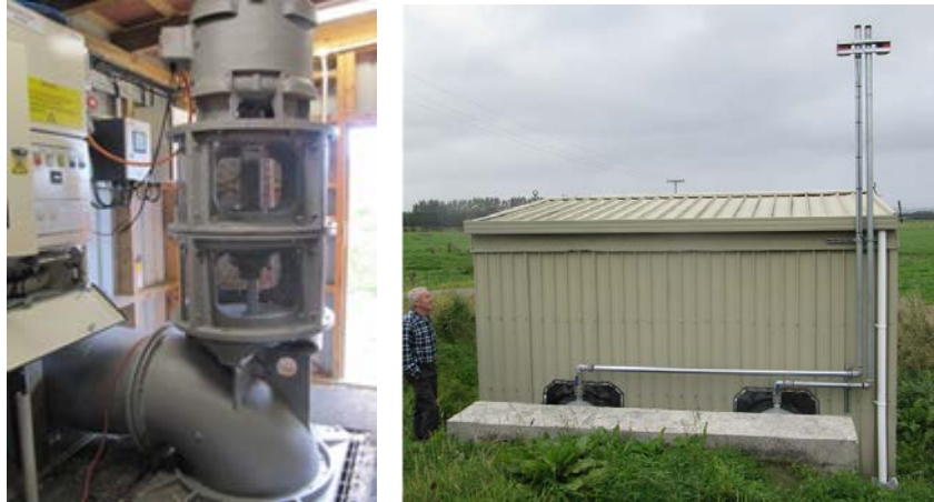
Figure 6: Smith Road Pump Station - Showing reconditioned pump, new piping, and new control cabinet.
