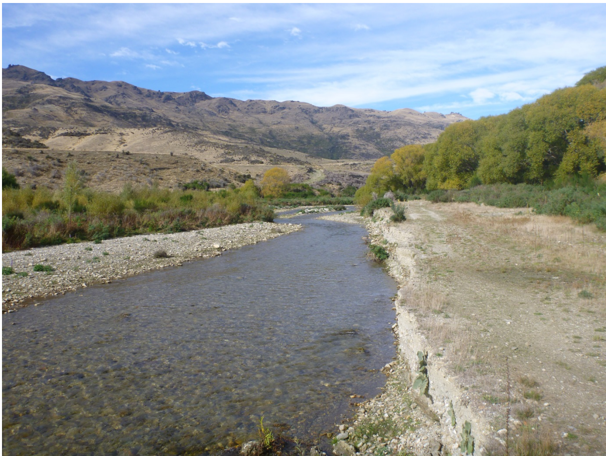
Figure 13. Bank erosion of the true left bank downstream of cross-section CR11-1 (Figure 6)
