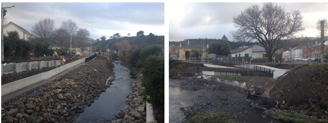
Figure 1: Dundas Street to St David Street Reach of the Water of Leith, St David Street pathway (left) and Dundas Street switchback pathway (right), on 30 June 2016, showing civil works largely completed.
