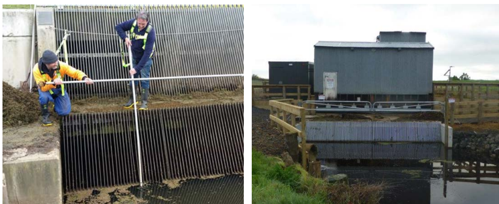
Figure 2: Weed raking trials at Waipori Pump Station (left). A gate arrangement to provide fall protection above an intake screen at a pump station in Waikato (right).
