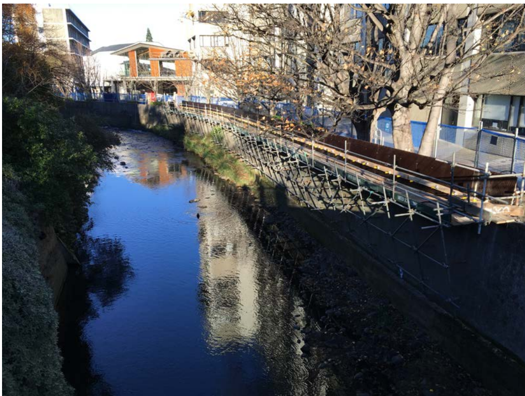
Figure 2 Water of Leith right bank wall raising works. Starter bars have been installed along the top of the existing wall in preparation for raising the top by approximately 600mm.
