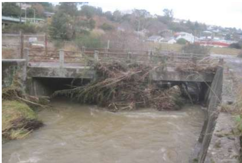
Figure 36. Tree and debris trapped under bridge at Burnside, 3 June 2015
