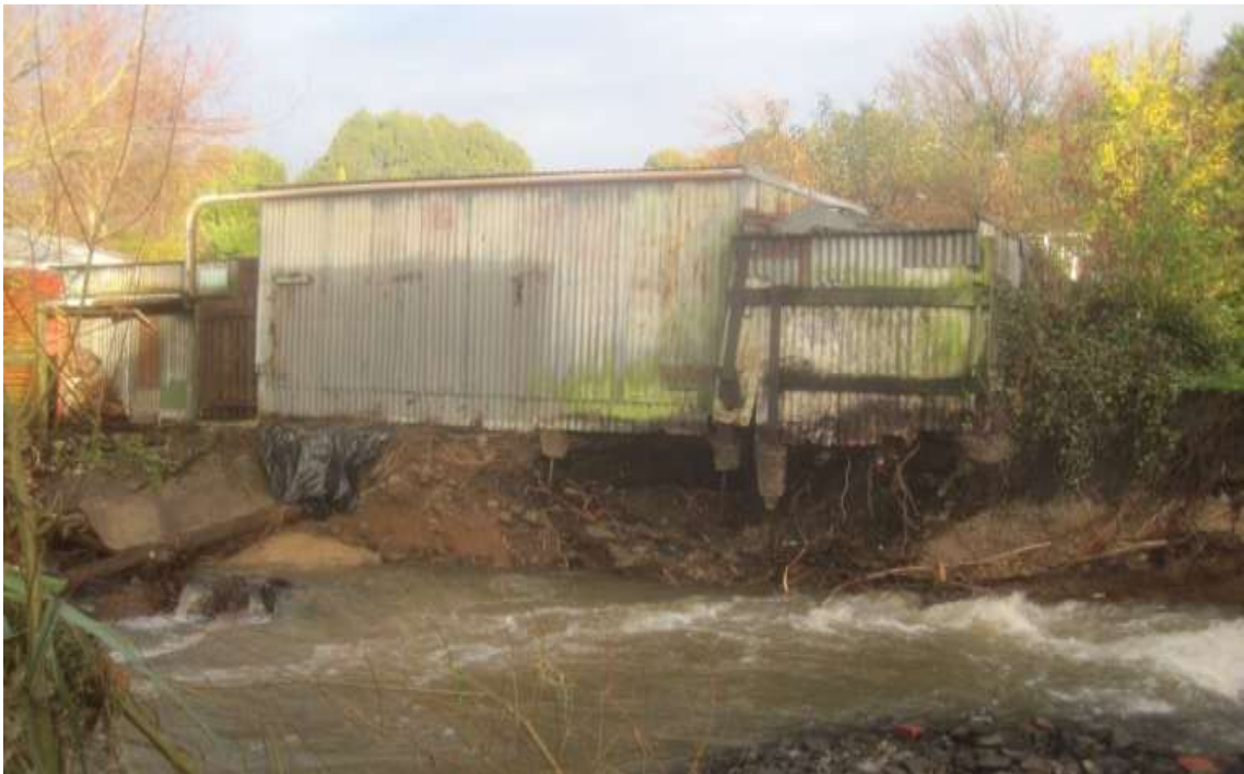
Figure 30. Bank erosion undermining a shed alongside Lindsay Creek at Kelvin Road, 4 June 2015
