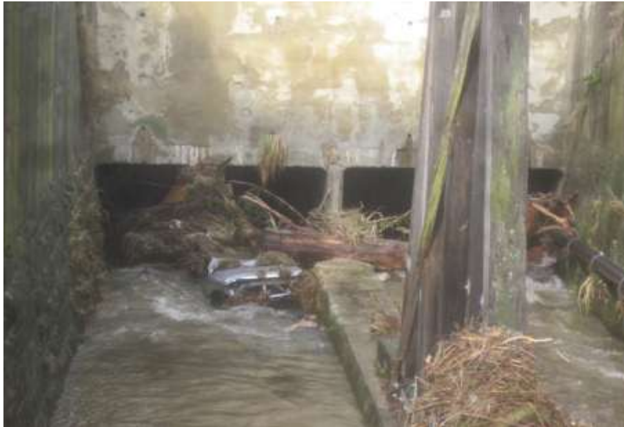
Figure 35. Car and tree lodged in culvert beneath SH1 at Burnside, 3 June 2015
