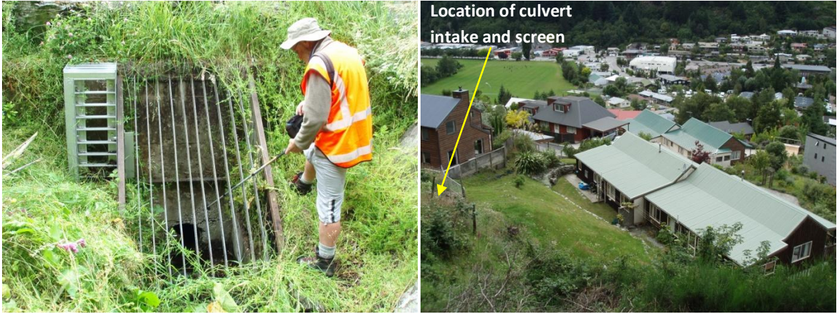
Figure 11.5 Reavers Lane alluvial-fan stormwater screen and culvert entrance (left). Residential properties at the head of the alluvial fan with respect to location of this structure (right)
