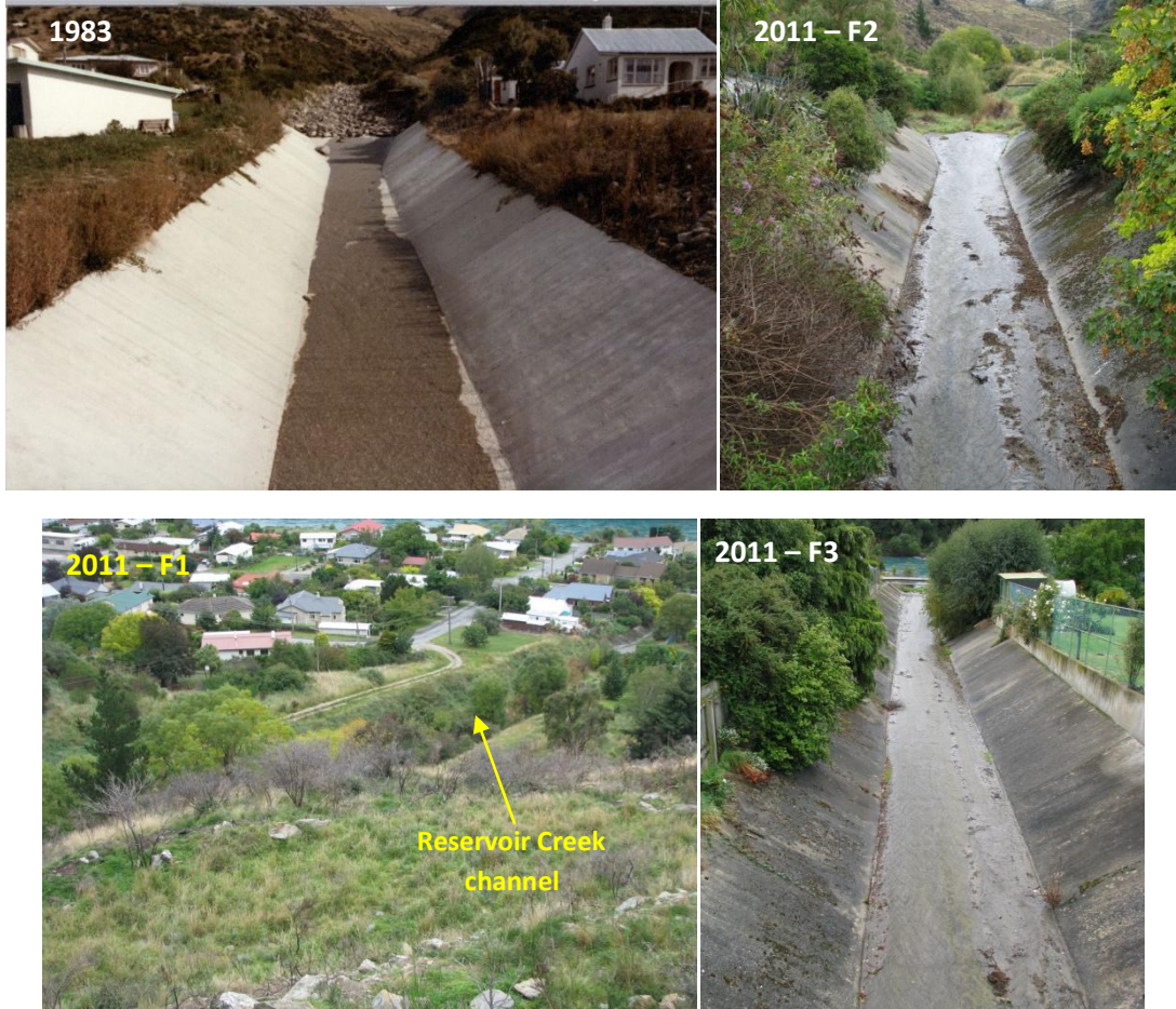
Figure 12.6 Reservoir Creek concrete-lined channel, upstream of SH 8 in March 1983 (top left), and in March 2011 (top right), looking upstream. Bottom left: Reservoir Creek channel upstream of concrete-lined channel. Bottom right: Reservoir Creek concrete-lined channel below SH 8
