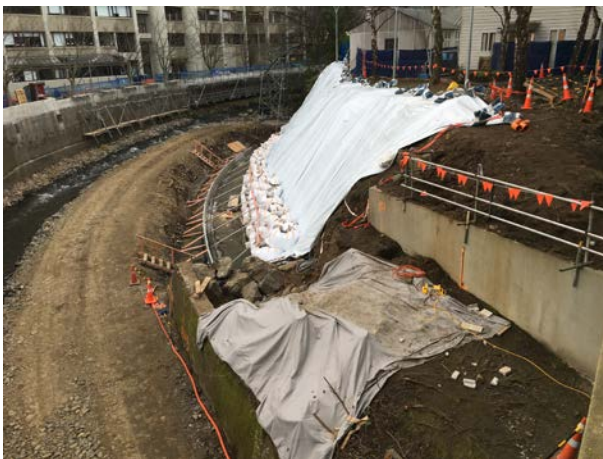
Figure 4: Leith Flood Protection Scheme works underway on left bank between Union Street and Leith Footbridge on 24 August 2017
