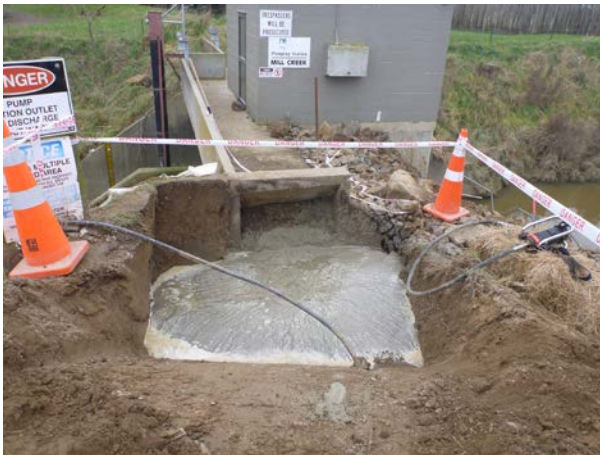
Figure 2: Mill Creek pump station (East Taieri Drainage Scheme) with temporary repairs underway to reduce risk of further seepage and piping
