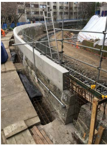
Figure 3: Leith Flood Protection Scheme works underway on right bank between Union Street and Leith Footbridge on 21 August 2017 (top) and 24 August 2017 (bottom).
