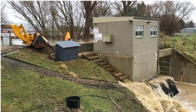
Figure 1: Seepage flow around Mill Creek pump station (East Taieri Drainage Scheme) on 22 July 2017
