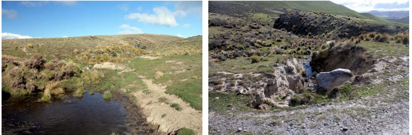
Figure 22 Left: Pond in the middle reaches of Deepdell Creek tributary. Right: Erosion around downstream end of culvert from pond.
