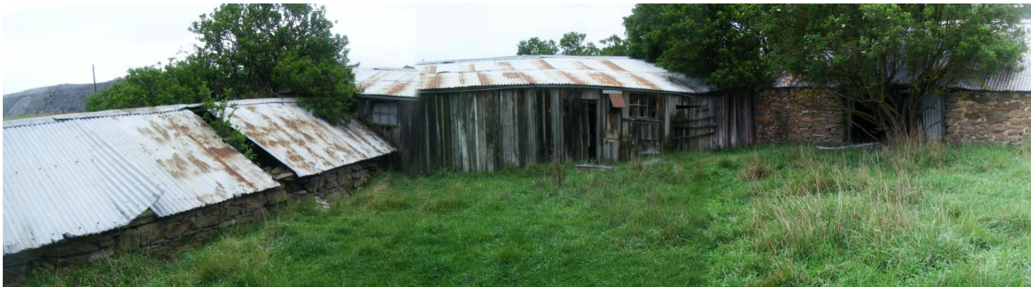
Figure Twenty Five Merged photo showing a general view of central yard of woolshed complex. Shed on left, shearing shed in centre, shed on right
