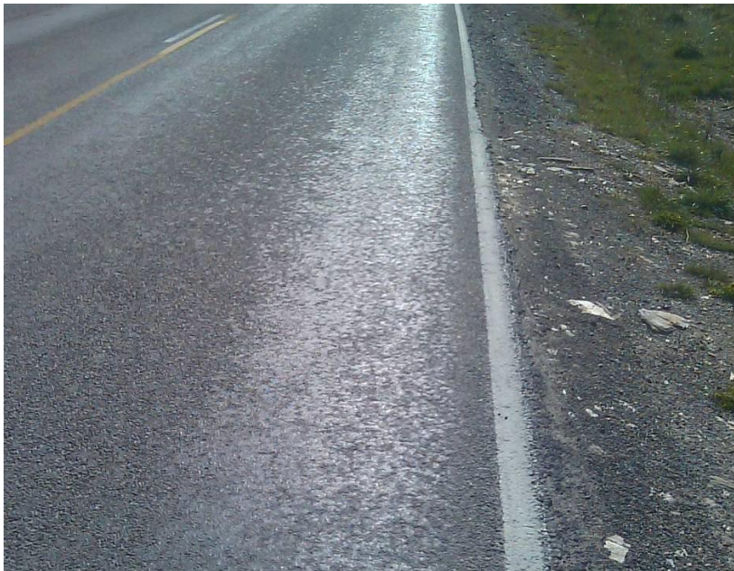
Photograph 6: Tar bleed and edge breakage on Macraes Road east of Macraes Road / Golden Bar Road intersection
