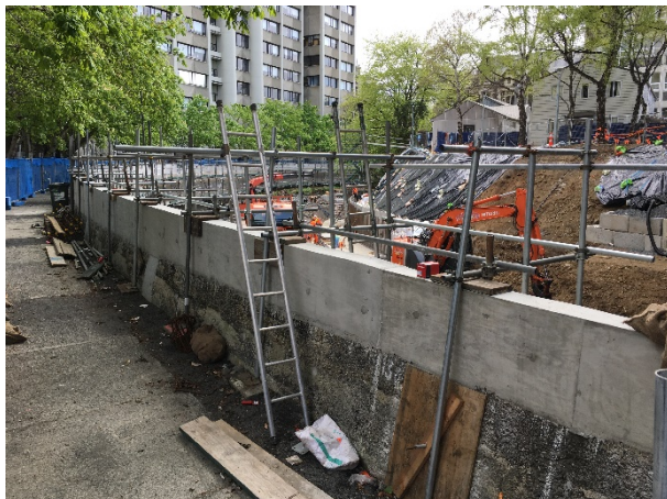
Figure 2: Leith Flood Protection Scheme works underway on right bank between Union Street and Leith Footbridge on 9 October 2017.
