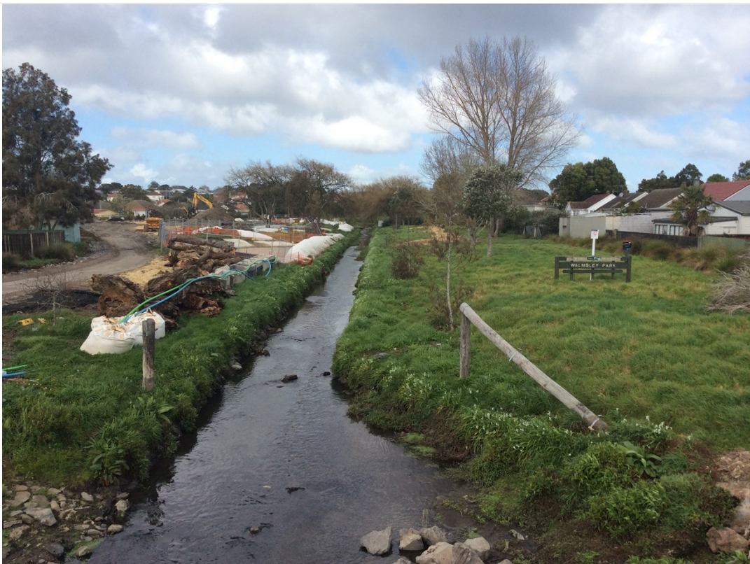
Figure 6: Restoration of Oakley Creek, Auckland. Restoration works underway in one section (top) and about to commence on another section (bottom).
