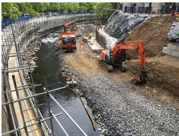
Figure 3: Leith Flood Protection Scheme works underway on left bank between Union Street and Leith Footbridge on 9 October 2017.
